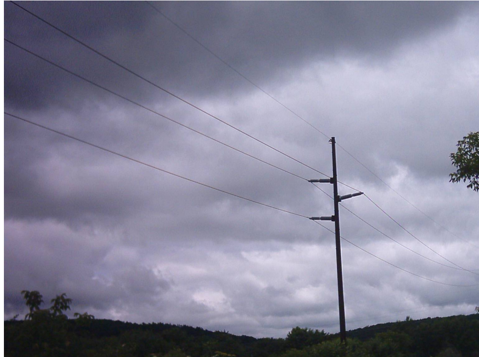
Figure 2. 115-kV transmission line in delta configuration at Site 1.
