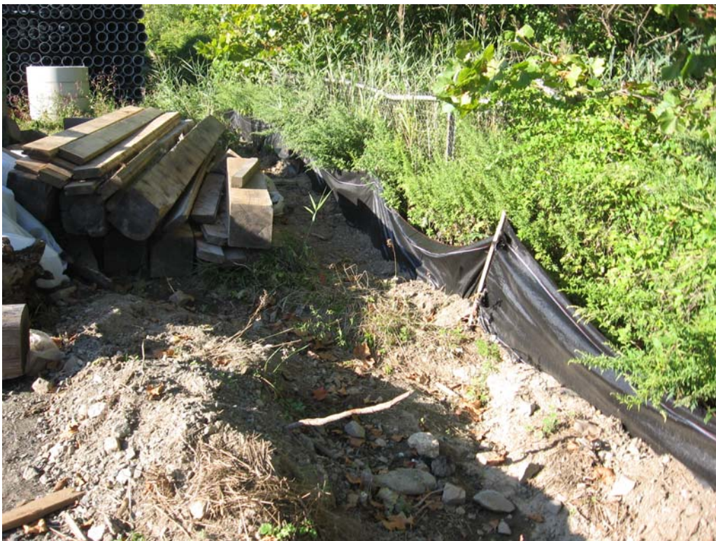
Photograph of erosion controls located adjacent to the watercourse within the King's Highway lay-down yard. Controls were formerly overwhelmed by materials, but have been re-established.
