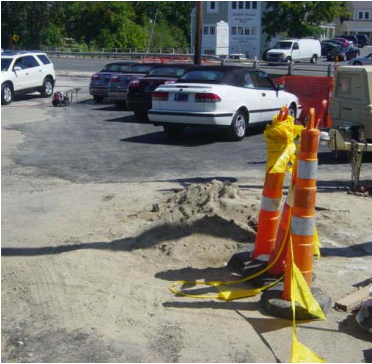
Photograph taken at sta. #217, adjacent to Stony Brook. An uncontained pile of sand was observed within the parking area.
