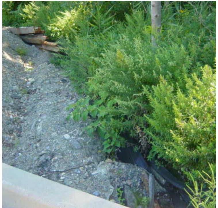
Erosion controls within the King's Highway lay-down yard remain compromised.
