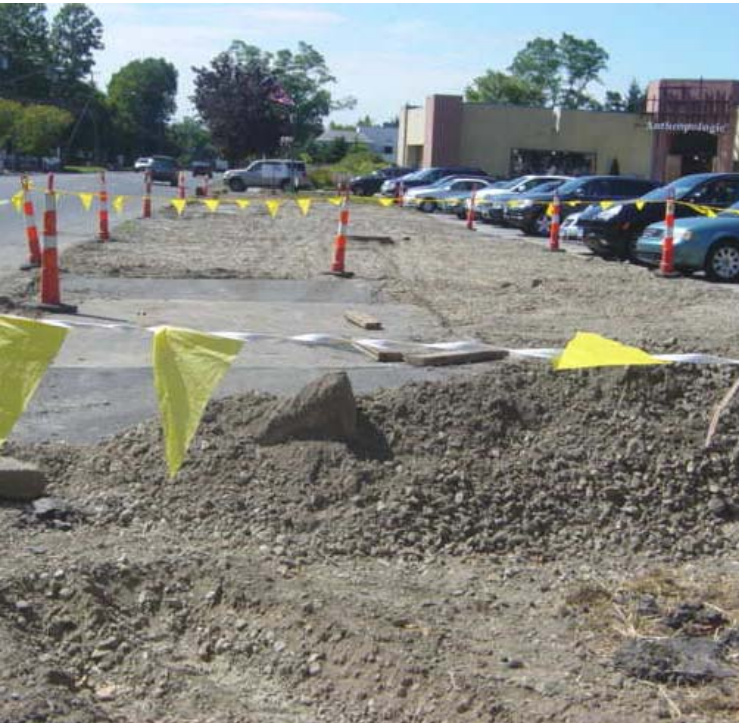
A hard packing material covers the work area at vault #23. Continue to monitor to ensure material does not migrate from the construction area.
