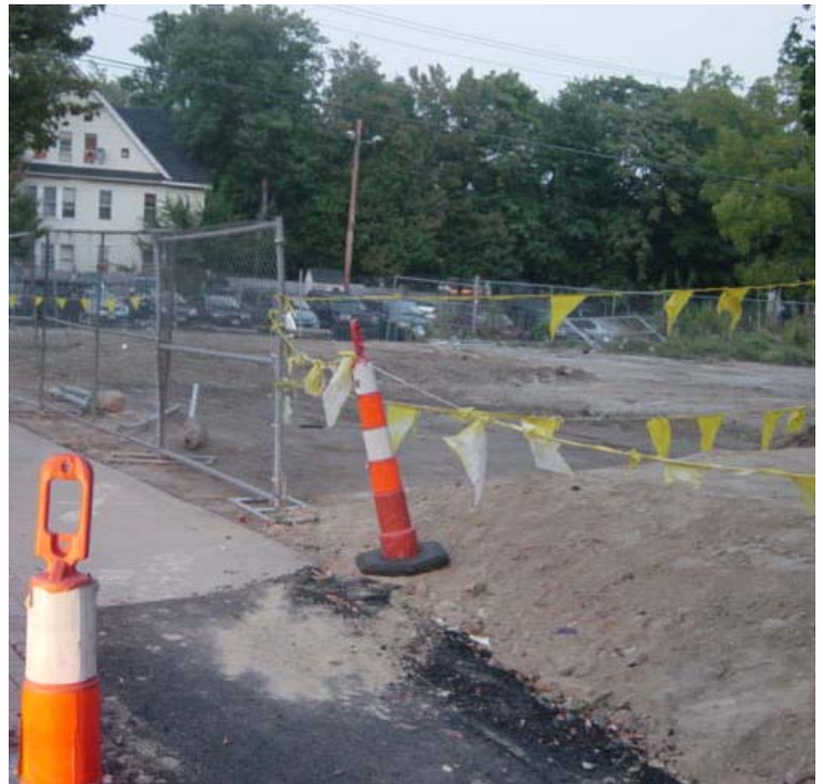
Utility work near sta. #695 has left soils exposed. It is recommended that exposed soils be stabilized or contained to prevent sediment migration.
