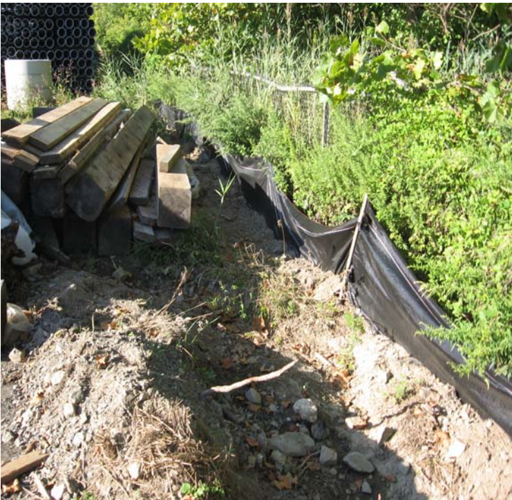
Erosion controls adjacent to the watercourse within the King's Highway lay-down yard have been re-established.
