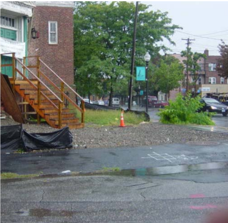
Compromised erosion controls at vault #41 have been removed.
