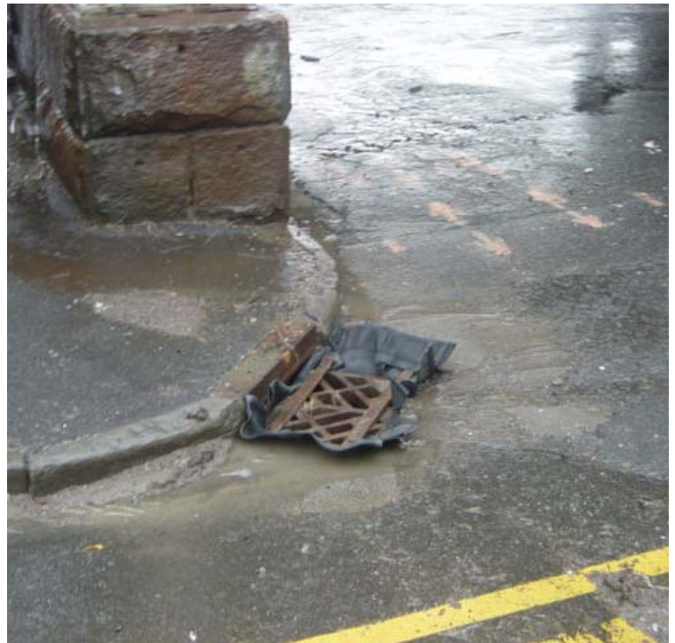
A number of silt sacks have been replaced along Railroad Ave. A few still require cleaning/replacement.
