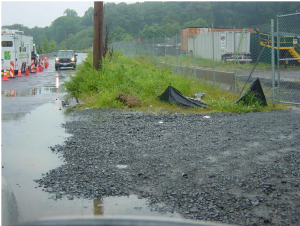
Non-project related debris remains just outside the entrance to the Milford yard and the stone construction entrance has migrated into roadway.
