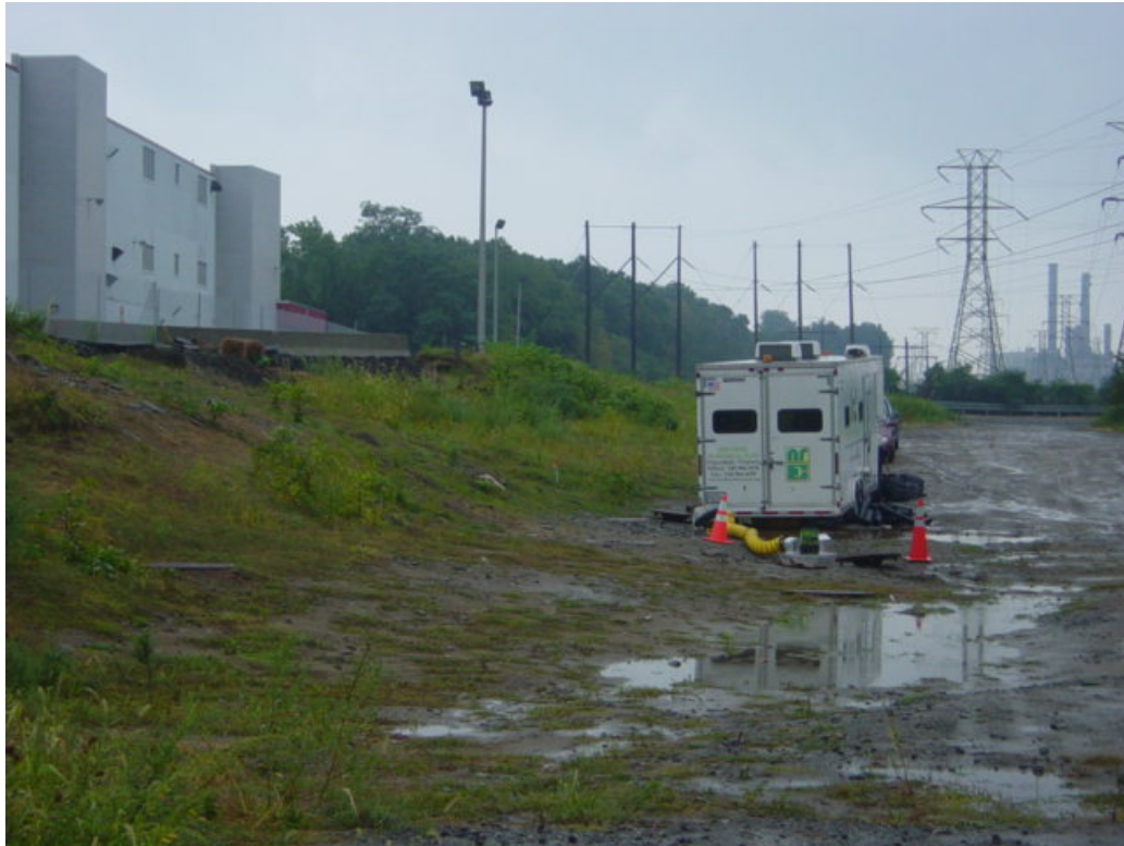
Photograph of electrical work at vault # 5 during heavy rains. Partially exposed slope remains stable.
