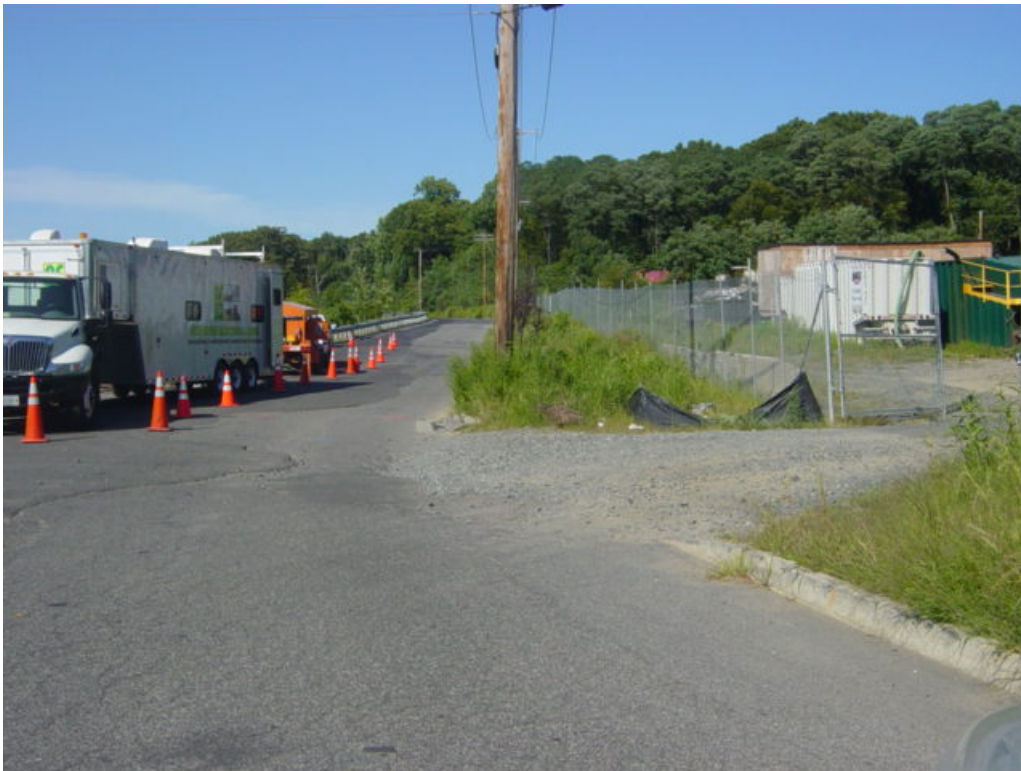
Photograph of the electrical work at vault #6 (left) and the Milford Lay-down yard stone construction entrance (right). The stone entrance has migrated into the roadway.
