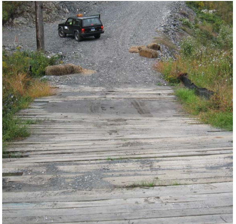
Litchfield Turnpike: Sediment should be cleaned from the timber mats as soon as possible and removed from the wetland when mats are lifted.
