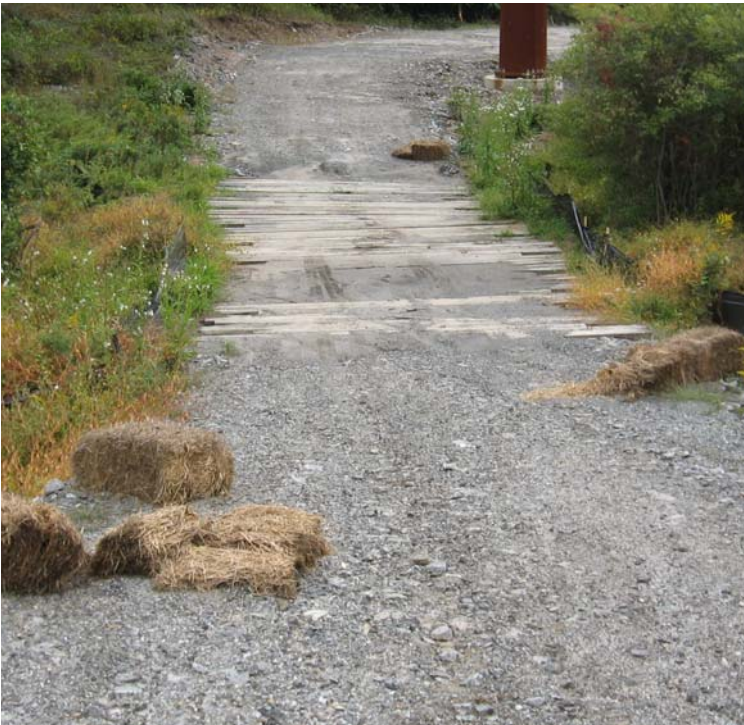
Litchfield Turnpike (Bethany): Additional controls are needed where sediment from the access road has migrated into the wetland.
