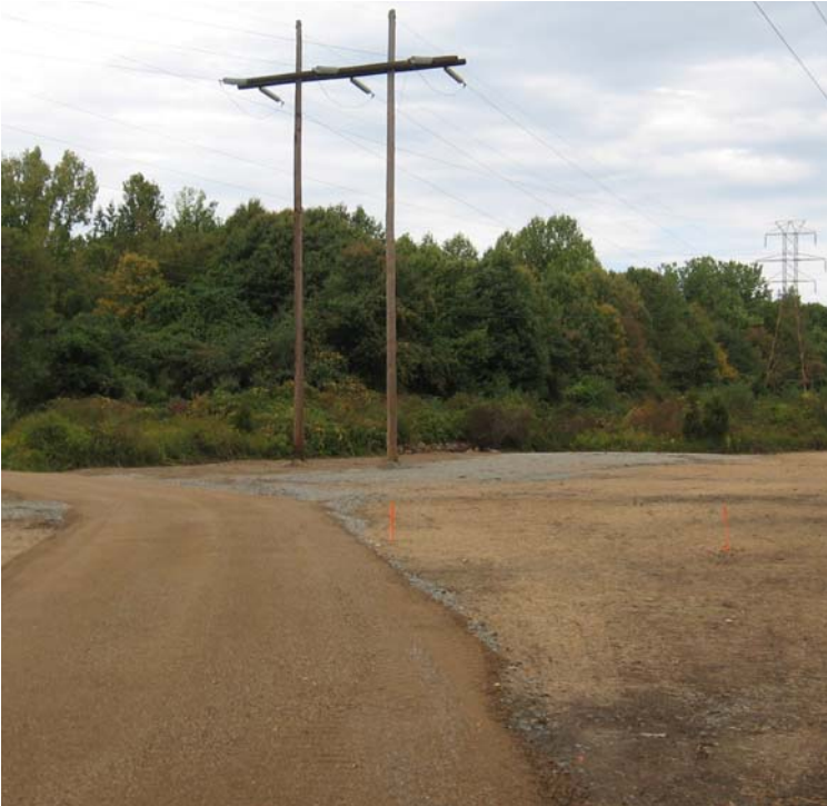
Eisenhower Park (Milford): Pad Reclamation and access road upgrades are complete in this area.
