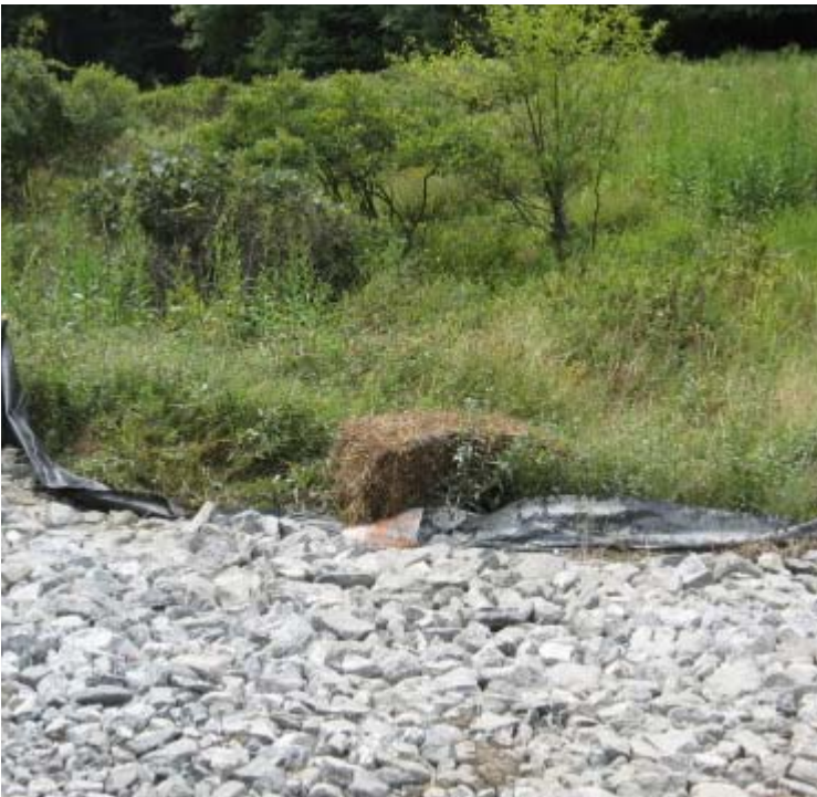
Clearview Lane to Route 15 (Woodbridge): Silt fence is in need of repair at structure #3903.
