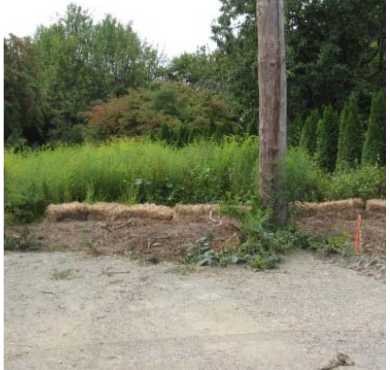
Hall Dr. (Orange): Pad reclamation activities continue. Additional erosion controls are recommended along the wetland boundary here.
