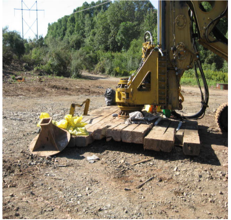
Durham Rd: Leaking equipment was noted here this week. Proper spill controls were in place.
