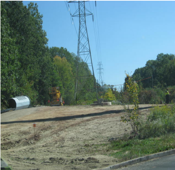
Old Farms Rd: Exposed soils were hydroseeded, but some ruts were noted here.
