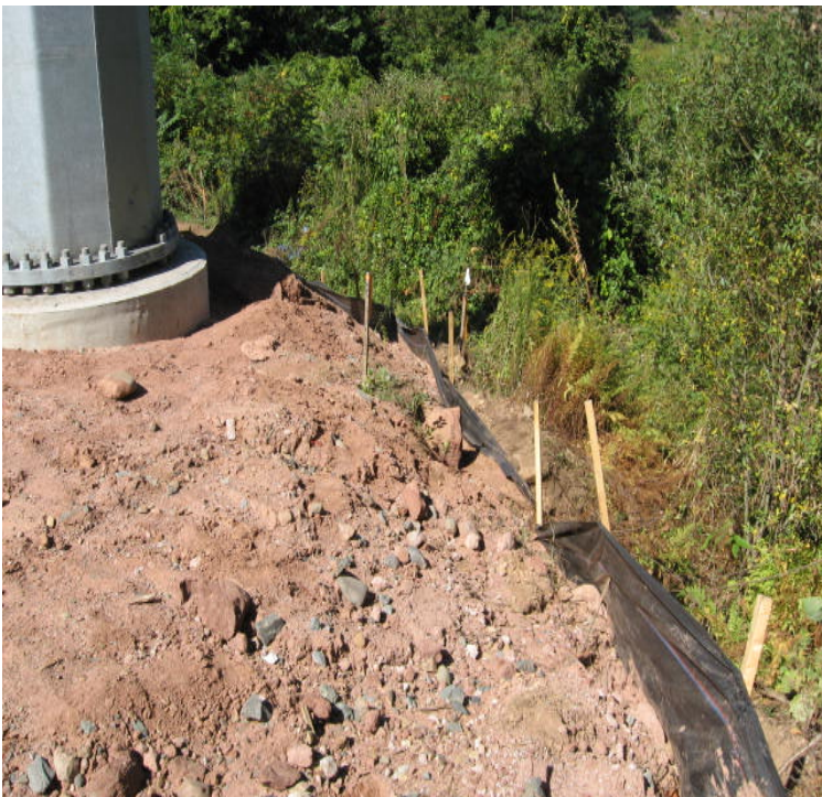
Docker Dr: Exposed soil resulting from recent foundation work has overwhelmed controls near the wetland here.
