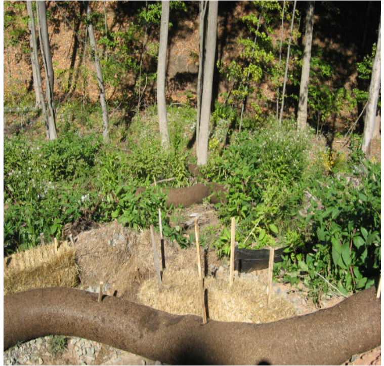
Harrison Rd: Haybales and a silt sock are in place at the sediment trap and along the slope.
