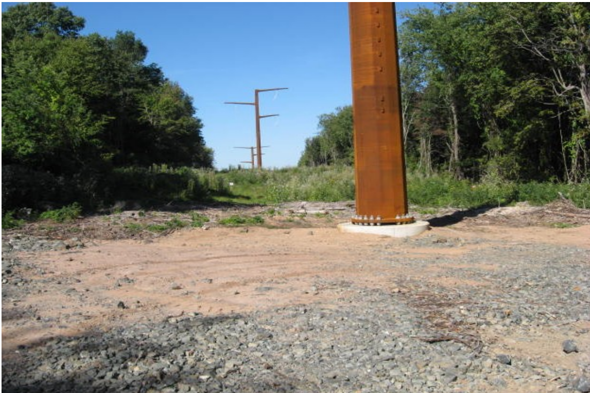
Sediment was observed at the edge of the no access area near the receiving yard. Continue to monitor and add controls as needed.
