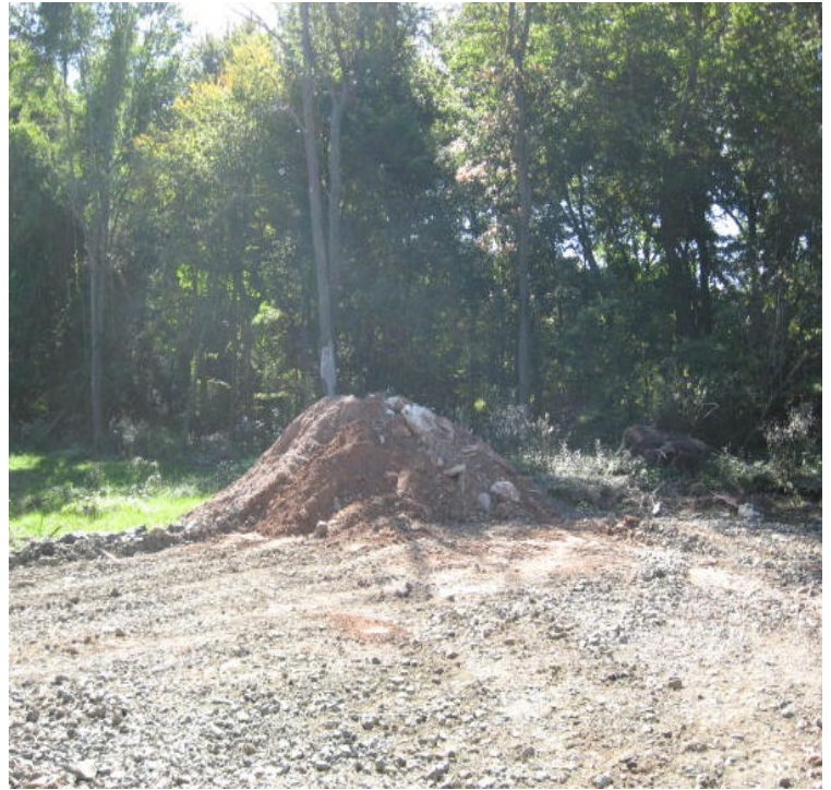
Soil stockpile noted near Black Walnut Dr. access. Remove pile or add appropriate controls.
