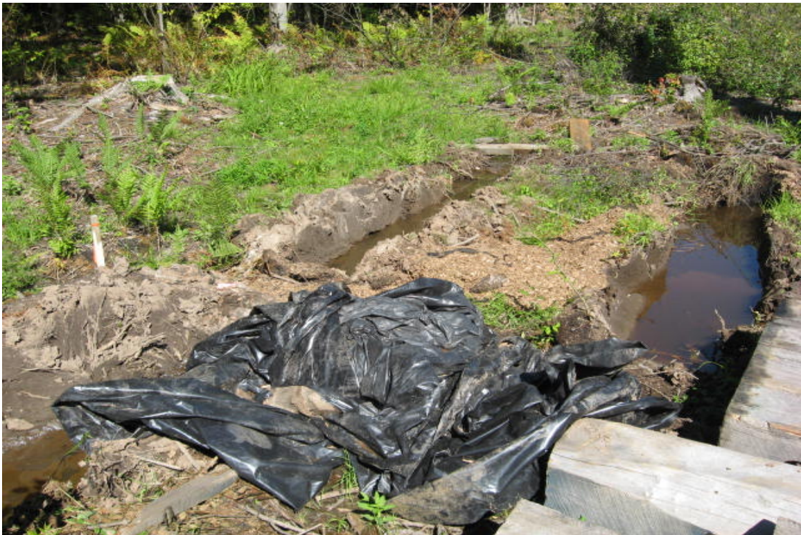
Equipment ruts were noted along the wetland edge within the no access area of Rte 17. Remove tarp from wetland and carefully regrade the ruts. Seed the disturbed area with a wetland seed mix.
