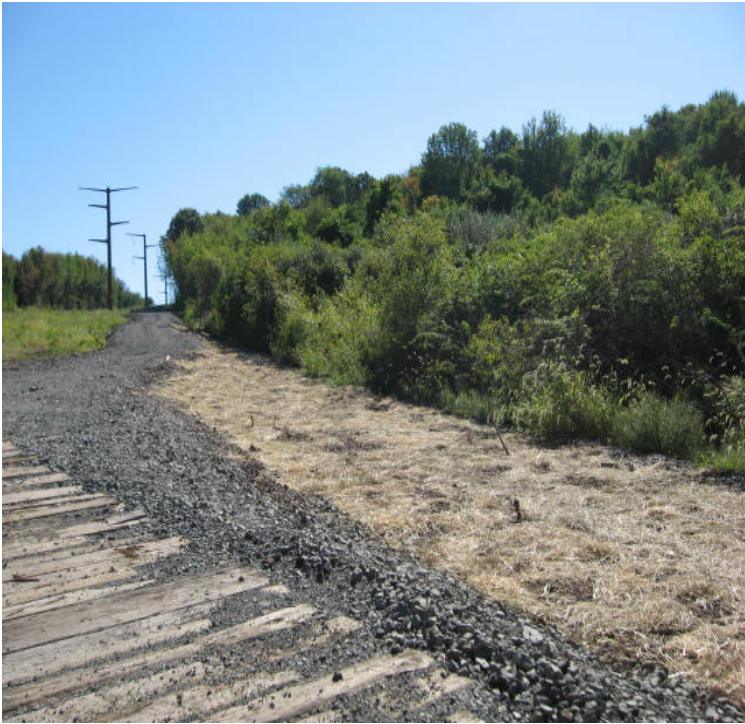
A section of the access road has been removed at Route 17 east. The disturbed area along the road was regraded, mulched, and seeded.
