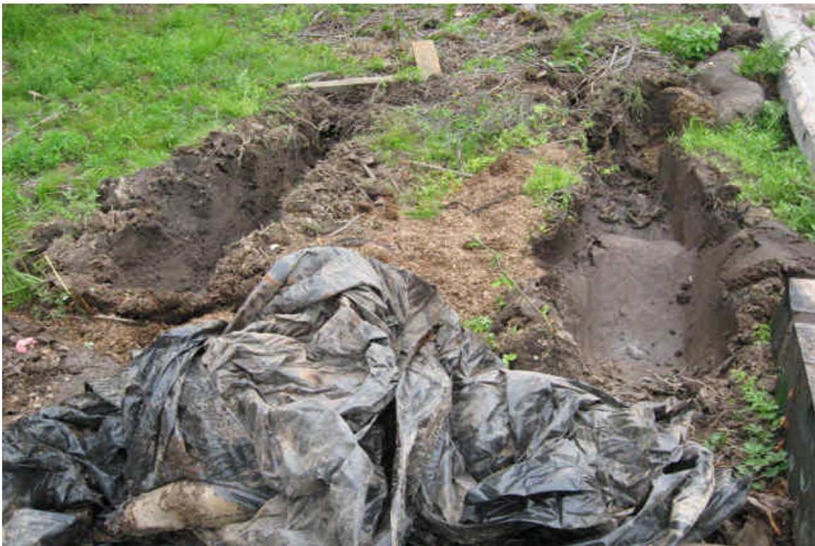
Looking across the no access area towards Little Lane. Some deep equipment ruts were noted at the edge. Carefully regrade the area and remove debris.
