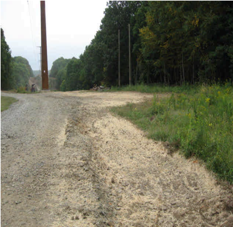
A section of the access road has been removed and graded. The area along the road was mulched and seeded.
