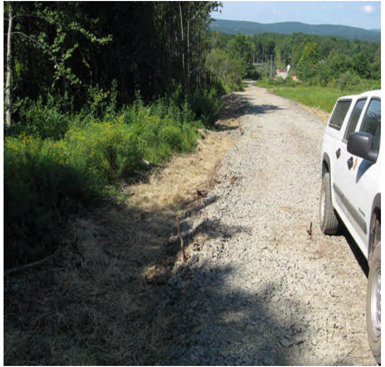
View of a drainage channel along the road with check dams, hay mulch and seed.
