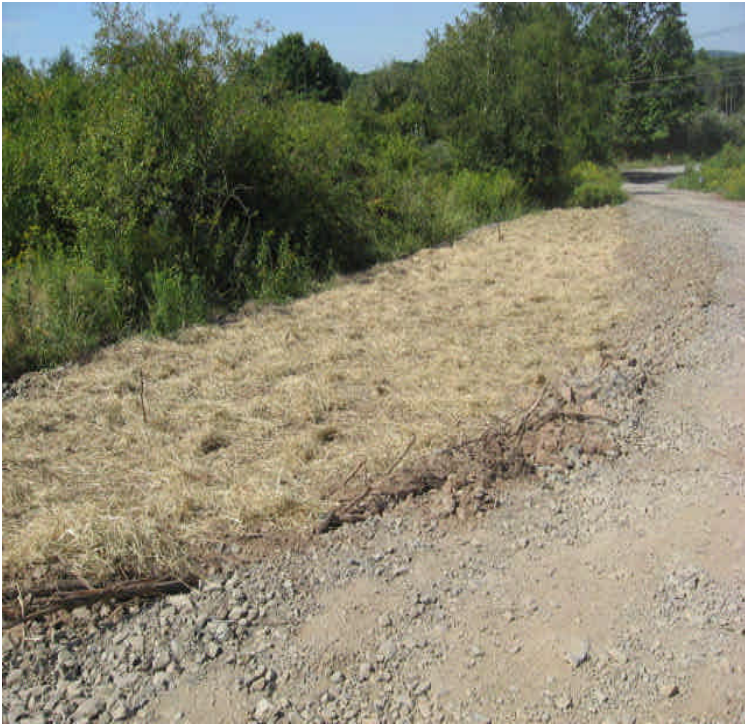
A portion of the access road has been removed and graded. The area along the road was mulched and seeded.
