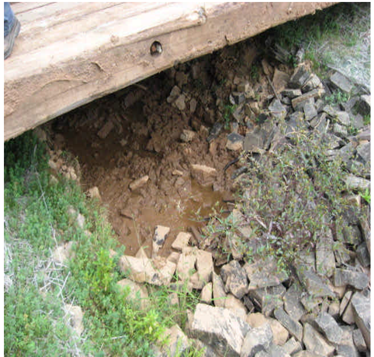
East Meriden SS (North): Timber mats were recently relocated and placed over the riprap stream bypass. This caused sediment to fall from the underside and accumulate in the channel.
