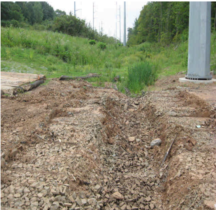
East Meriden SS (North): The original stream channel that had been filled/redirected for the work was carved out. Remove remaining fill and stabilize the adjacent areas. Remove the riprap bypass before accessing or working at the new pad site.
