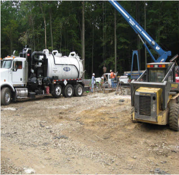
Shunpike Rd: Crews were dewatering a foundation and pumping into a settling tank for containment.
