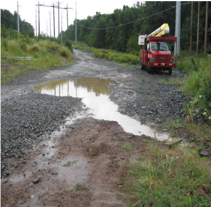
Carpenter Lane (north): Turbid water was noted flowing off-site during a heavy rain storm on 9/11/07.
