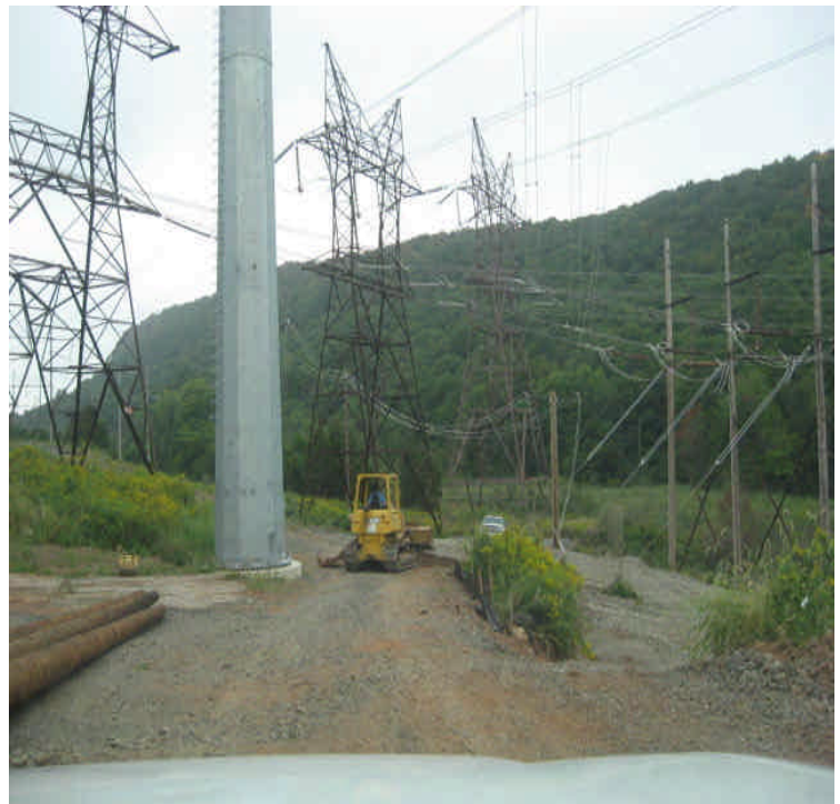
Black Pond Jct: New pad site is in place at the edge/within wetlands.
