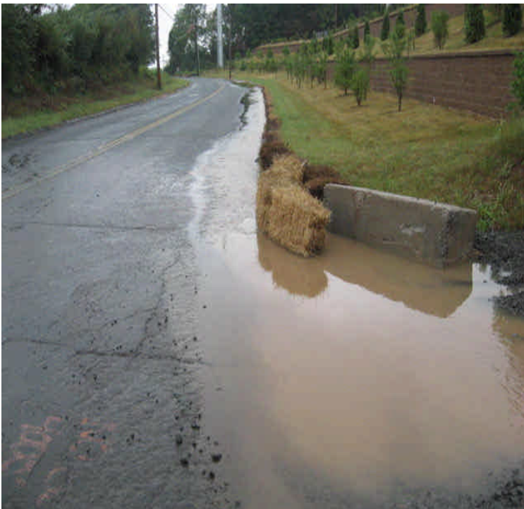
Turbid run-off at the eastern site access during the storm which brought over 1-inch of rain. Despite all the stabilization measures, exposed soil is still creating run-off issues from the site. If 1A contractors are creating stockpiles, as part of their work, they will have to be part of solutions here.
