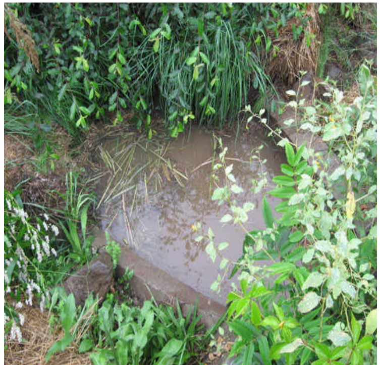
Turbid water starting to fill the storm drain across Carpenter Lane.
