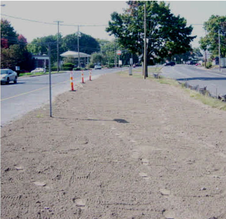
Topsoil has been spread near sta. #316-318. Seed and mulch is still required for stabilization of exposed soils.
