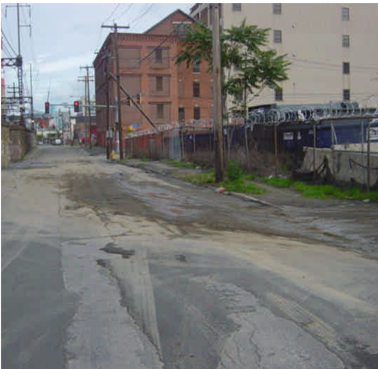
Heavy sediment tracking was evident along the roadway near the storage yard at Railroad Ave. and Myrtle Ave., associated with the Glenbrook Cable project. The down gradient catch basins remain protected with silt sacks. Although this area overlaps the M/N project route, it is not M/N project related.
