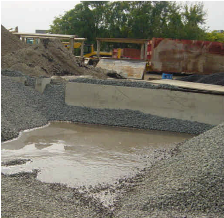
Concrete slurry washout had been performed within a contained stone stockpile area in the Kings Highway lay-down yard. Eventually, the material should be removed and properly disposed of.
