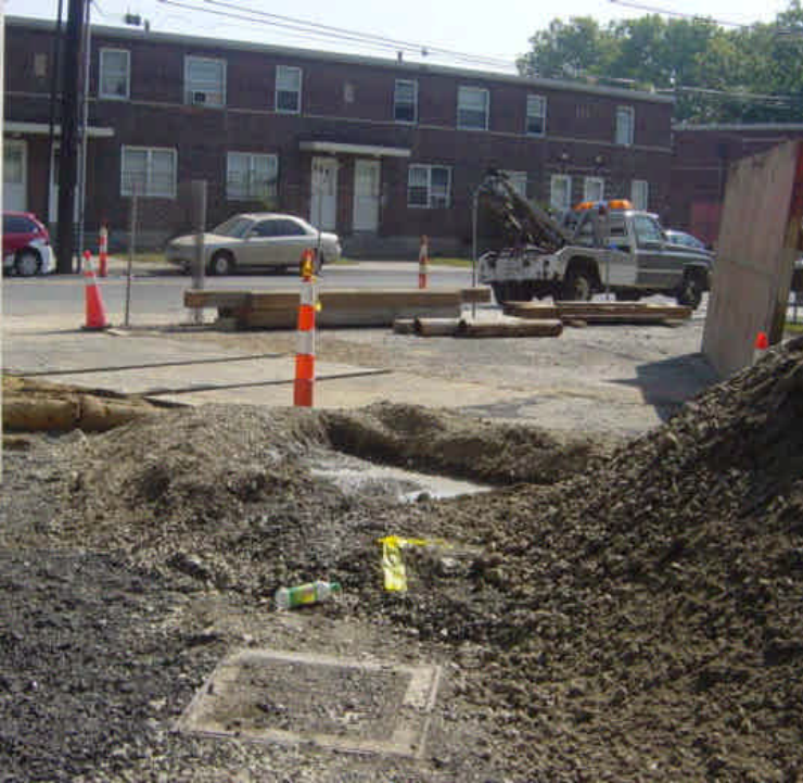
A small, designated concrete washout area was observed near the trench work at Sta. #771-#772.
