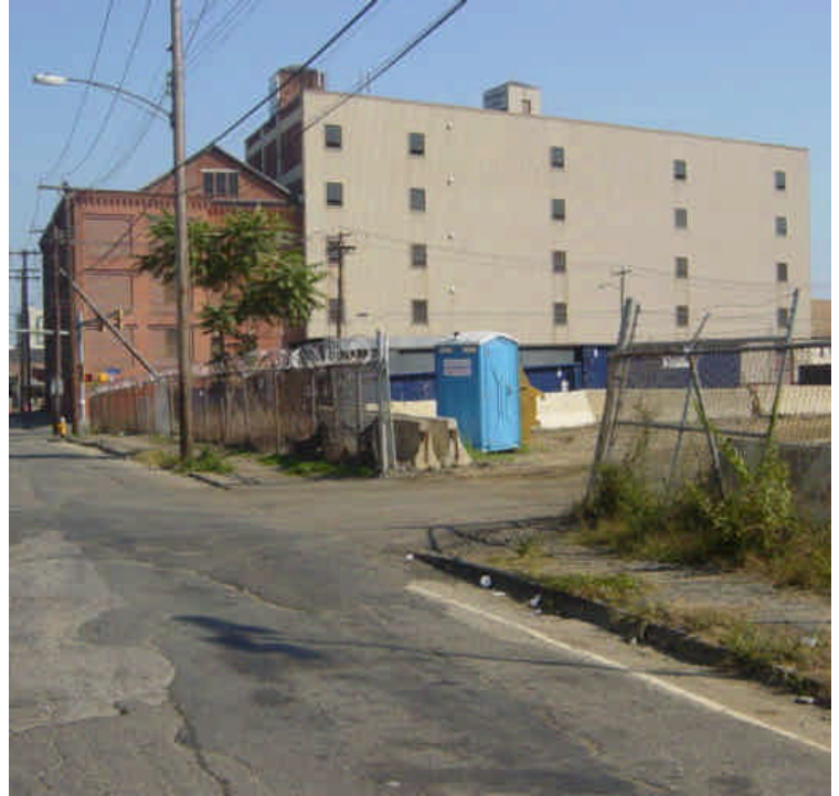
Calcium chloride was applied to exposed soils at the storage yard at Railroad Ave. and Myrtle Ave., associated with the Glenbrook Cable project in order to control dust. The downstream catch basins have been protected with silt sacks. (This area is not related to the M/N project but is located along a portion of the route.)
