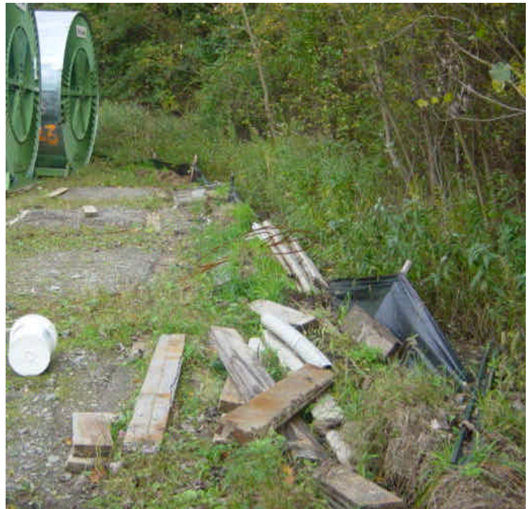
Sections of silt fence along the south side of the Shelland St. laydown yard is sagging. The area is well vegetated and the silt fence continues to function. This yard appears to be idle as work has shifted to other areas of the project.
