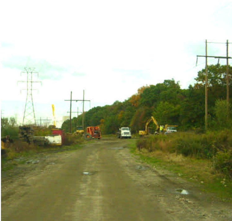
Work noted on the overhead lines along the cross country section between sta. #1051 to #1080 which overlaps the Segment 3 route.
