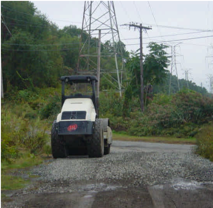
Equipment was being stored at sta. #1051 near the entrance to the ROW and less than 100' from the adjacent resource area. Equipment appears to be related to work on the overhead wires.
