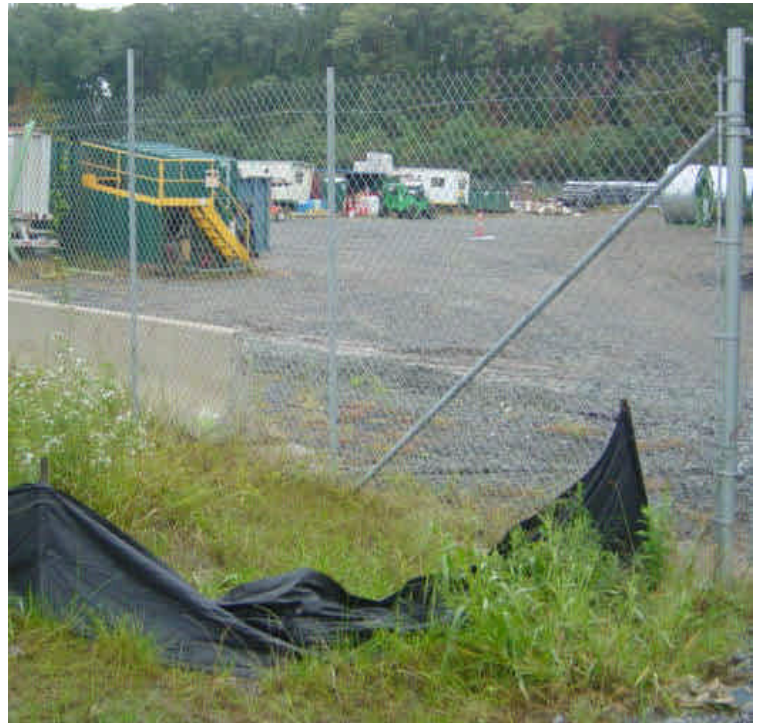
A small section of silt fence near the entrance to the Shelland St. laydown yard is sagging but continues to function. This yard appears to be idle as work has shifted to other areas of the project.
