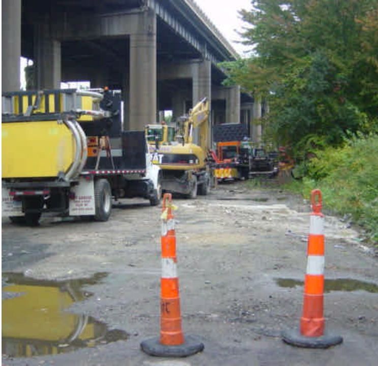
Construction activities that are not part of the M/N project have continued near sta. #1015-1020 (vault #1) for several months. This continues to disturb soil in the area and concrete washouts are a regular occurrence.
