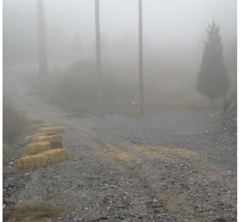
Litchfield Turnpike (Bethany): Haybale check dams have been installed along the access road to slow and filter stormwater flow, but further attention is needed here.
