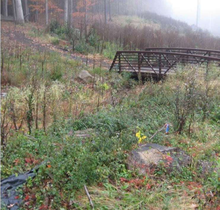
JCC (Woodbridge): Silt fence is in need of repair along the wetland boundary here.
