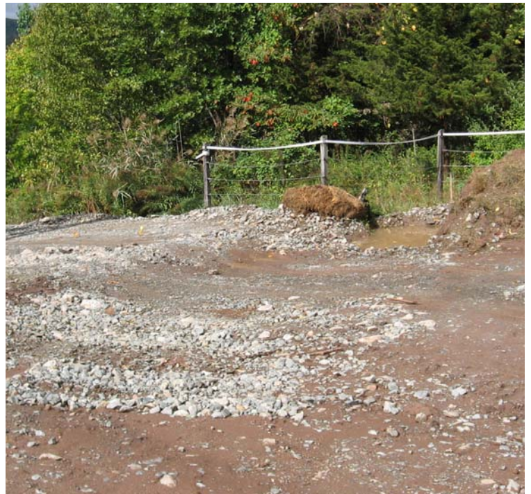
Old Lane Rd (Hamden): Storm water has been redirected from the access road to a haybale/silt fence check dam near structure #4013.
