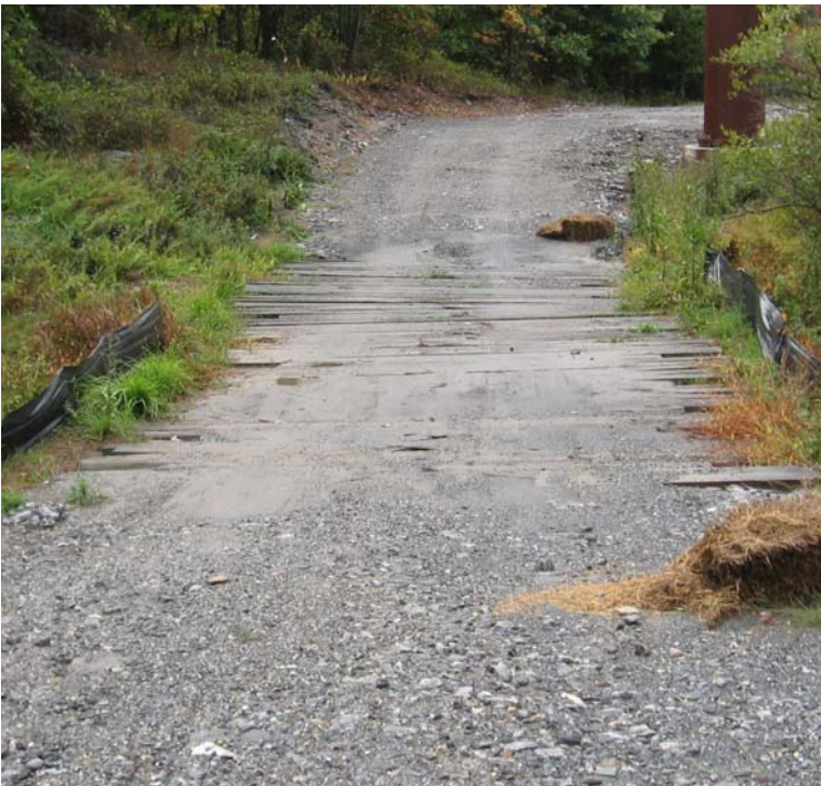
Litchfield Turnpike (Bethany): Excess sediment has accumulated on the timber mat crossings along the access road in this section. Sediment has seeped through the mats and into the wetlands at several crossings.
