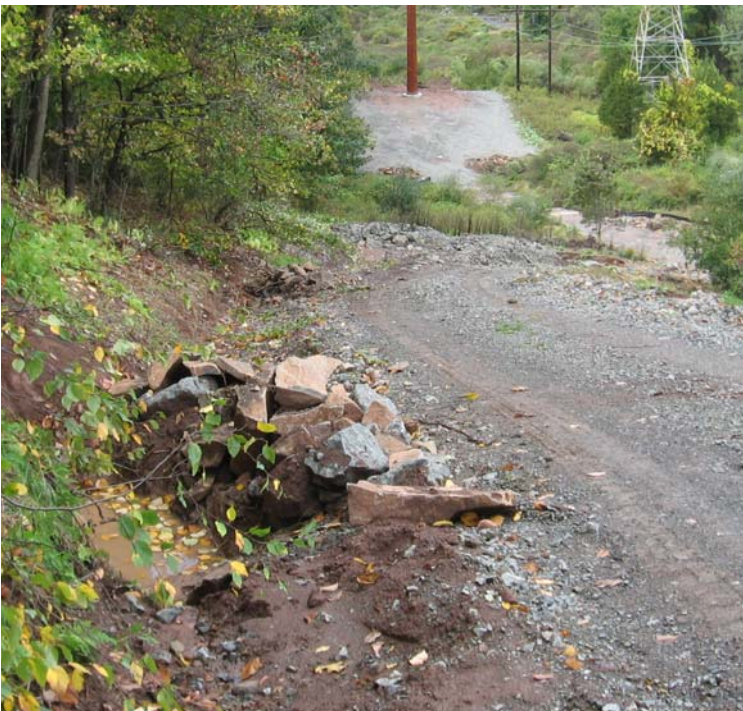
Old Lane Rd: View of the access road looking toward the stone sediment trap.
