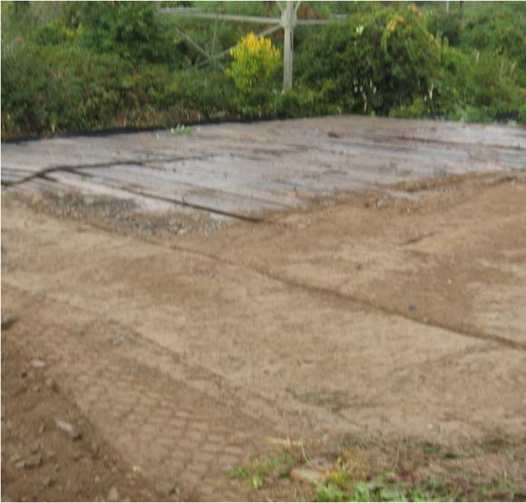
Naugatuck Ave (Milford): A timber mat crane pad was installed within the wetland at proposed structure #3804.
