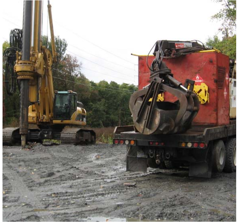
Pease Rd (Woodbridge): Drilling for the 345kV line has begun in this section.
