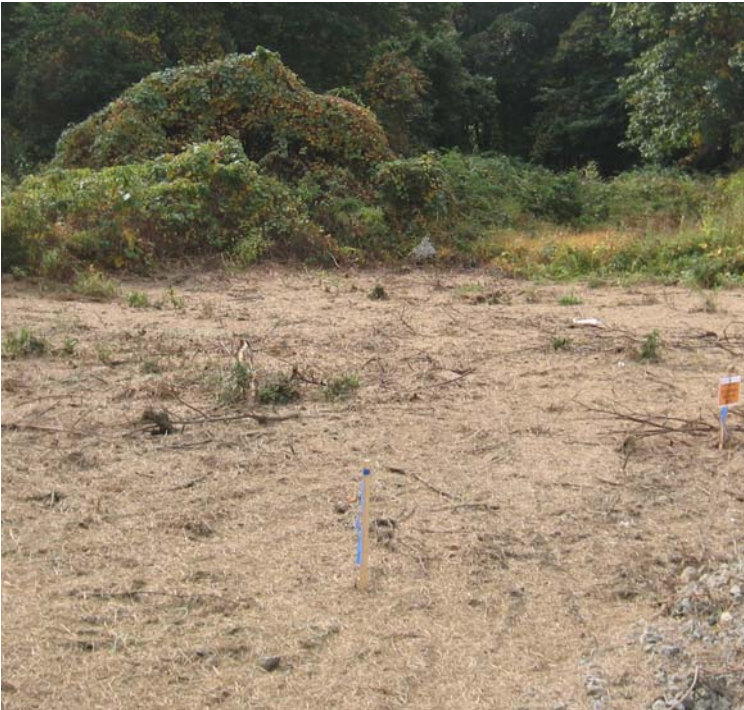
West River St: The timber mat crane pad has been removed and exposed soils have been graded, mulched and seeded at structure # 3838.
