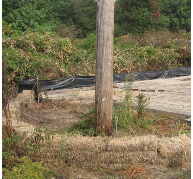
West River St: Pad reclamation is complete and proper controls are in place.
