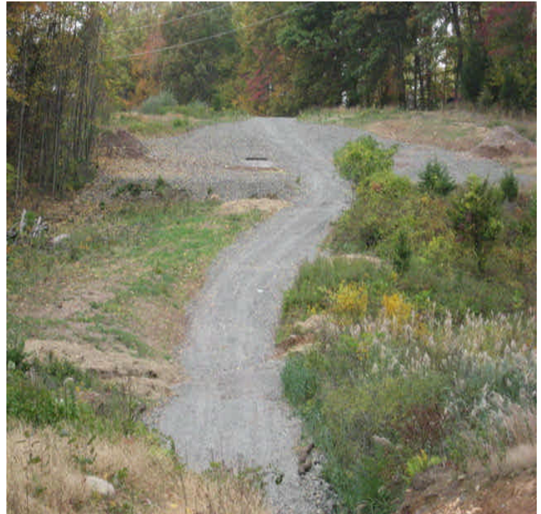
Tuttle Dr: Water bars were installed along the access road to divert stormwater into detention areas.
