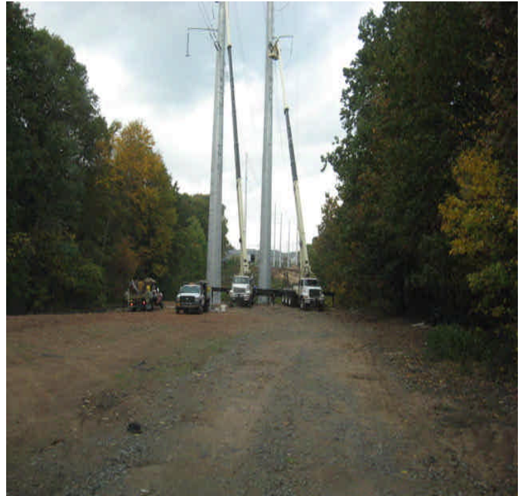
Docker Dr: Some exposed soils remain graded, mulched, and seeded. Crews were performing line work.
