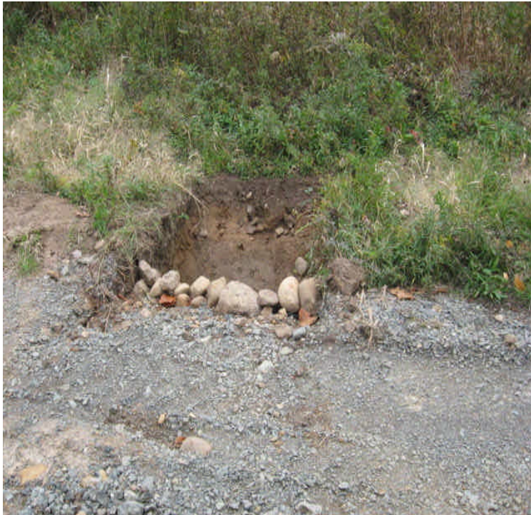
Mansion Rd Apple Orchard: Culvert was installed to reduce ponding on the access road.
