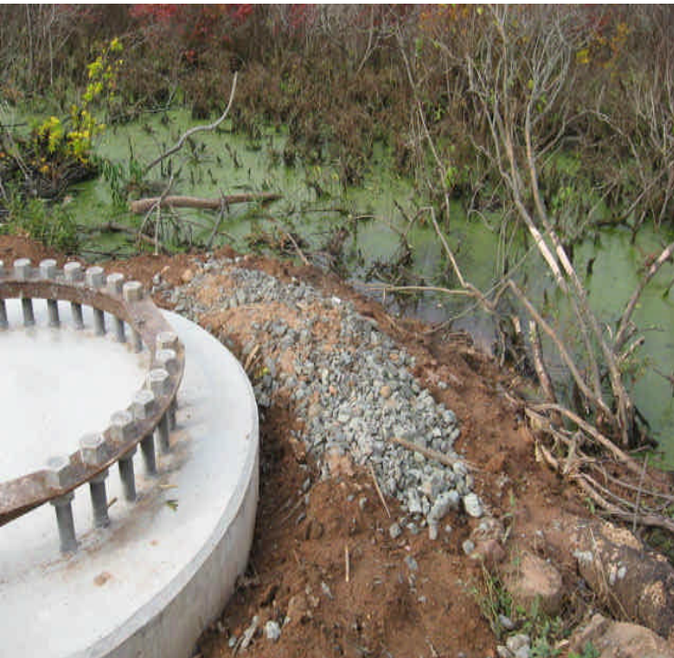
Tamarack Swamp Rd: Foundation was installed, but sediment was piled/pushed beyond the controls. Carefully pull sediment back and then reinforce controls. Avoid adding another layer of controls prior to removing the sediment.
