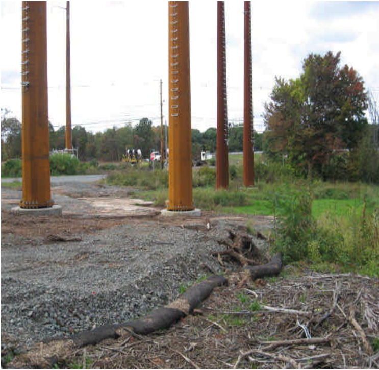
Powers Rd: Timber mats and stone/sediment were present within the wetland. Carefully remove sediment and reinforce controls.
