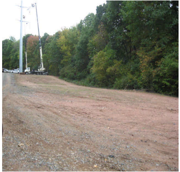
Docker Dr: Exposed soils remain graded, mulched, and seeded. Crews were performing line work.
