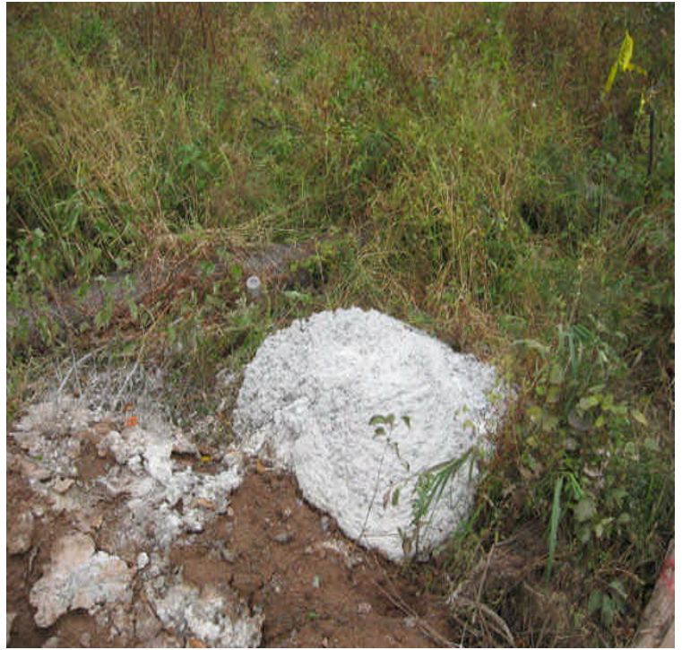
Liney Hall Ln: An excess concrete washout was noted within at the Wetland boundary.
