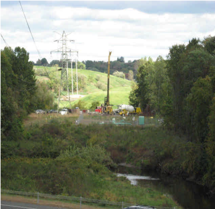
Pent Rd: View of foundation drilling underway at structure #24225, located between Wallingford landfill and the Quinnipiac River. This view also shows the extent of re-vegetation following the necessary clearing at the river.
