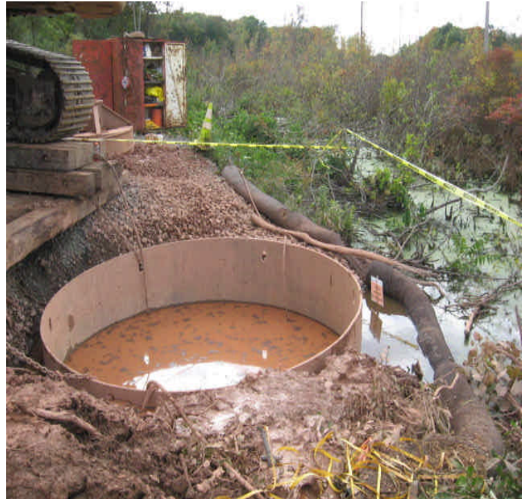
Tamarack Swamp Rd.: Foundation drilling and stockpiling the resulting sediment/spoil continues. Continue to monitor very closely and carefully contain the work due to the adjacent area of standing water.
