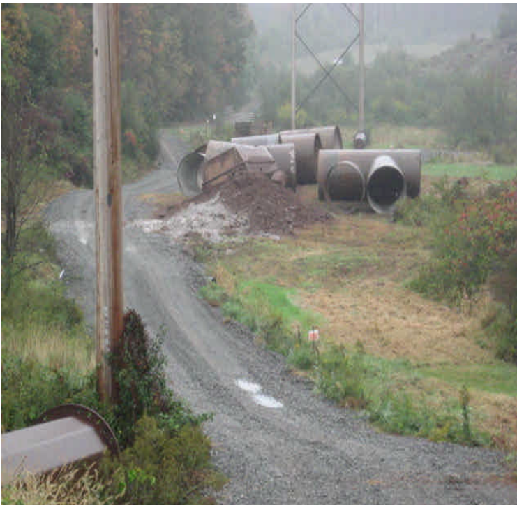
Liney Hall Ln: Soil stockpile and an uncontained concrete washout were noted upgradient from wetlands. It appears that there was an attempt to designate a washout area but it did not have adequate capacity.
