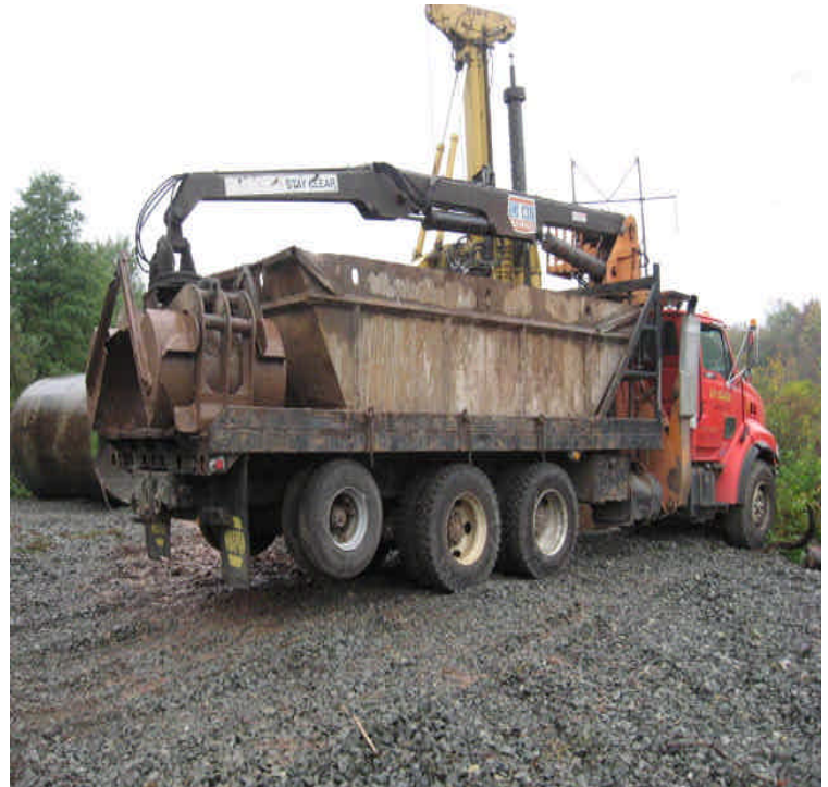
Tamarack Swamp Rd.: Foundation drilling and removal of the resulting spoil/sediment was underway.
