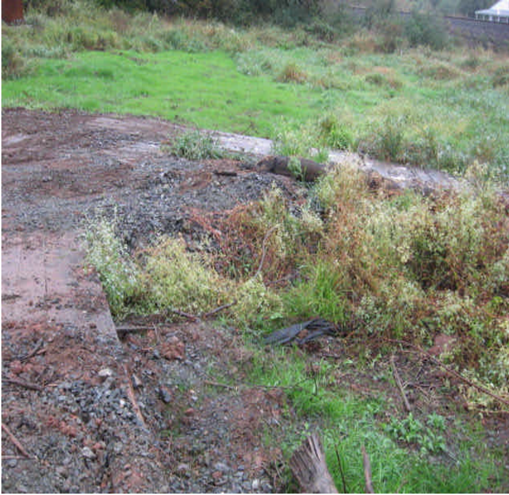
Powers Rd: Timber mats and stone/sediment were present within the wetland. Carefully remove sediment and add controls.
