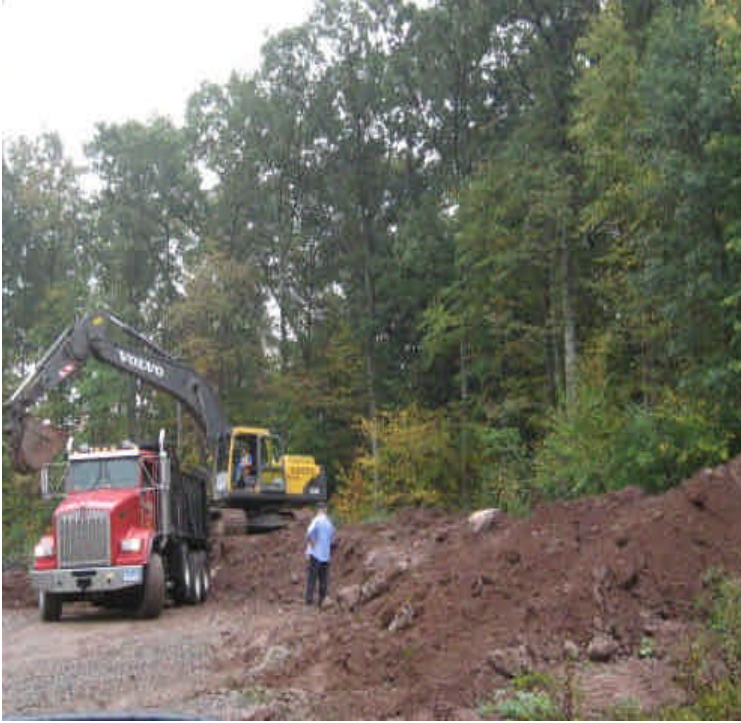
High Hill Rd: Foundation drilling and removal of resulting spoils is underway.
