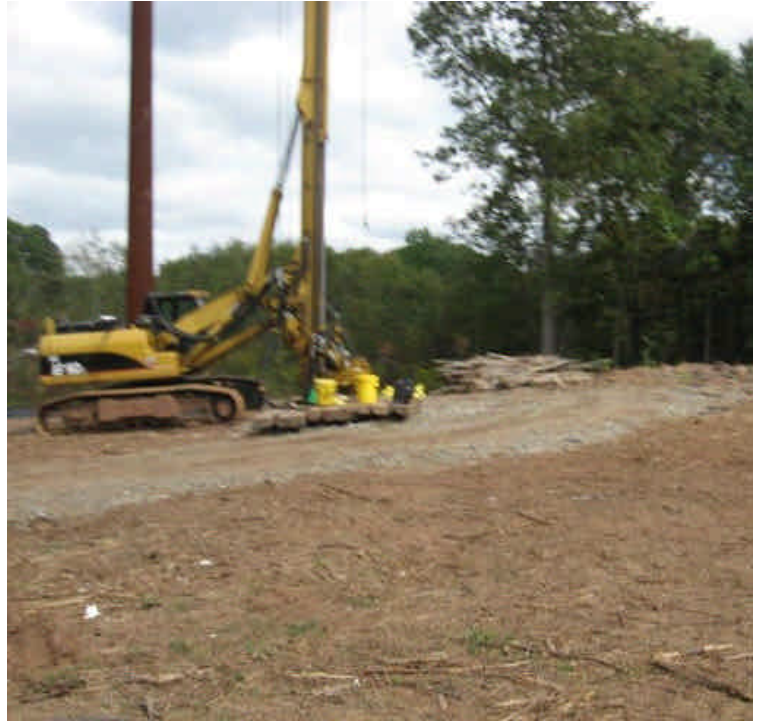
Durham Rd: View of leaking equipment with controls in place. Repair the equipment as soon as feasible.
