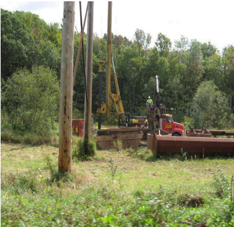
Liney Hall Ln: Crews were working within a wetland, drilling a foundation.
