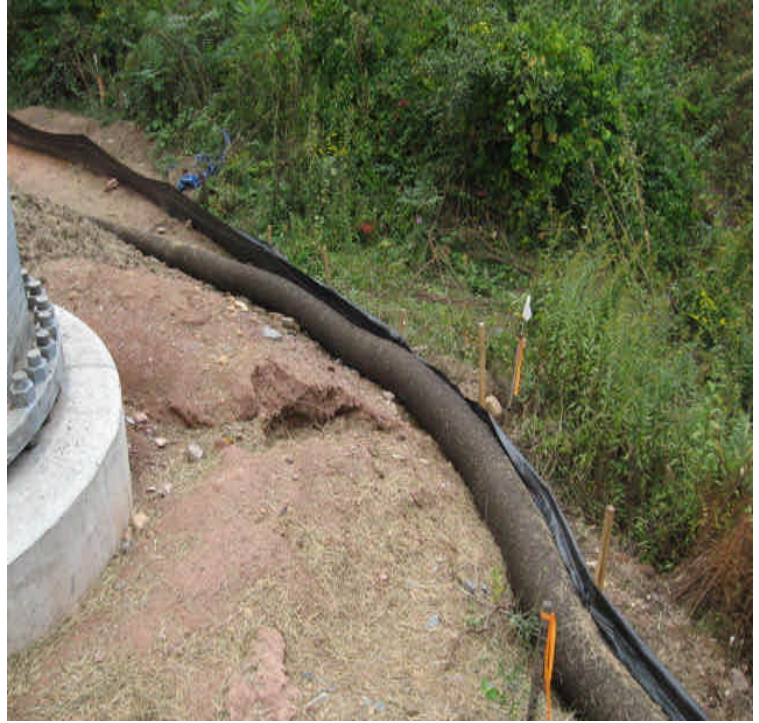
Docker Dr: A silt sock was installed upgradient from the wetlands at the new foundation where controls were overwhelmed last week. The disturbed area was mulched. Regrade and stabilize the small, eroded channel as needed.
