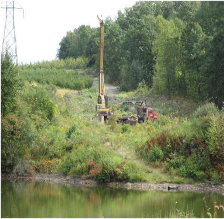
Orchard: Foundation drilling was occurring within the apple orchard, upgradient from the wetlands.
