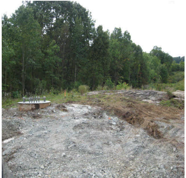
South Turnpike: Disturbed area remains at the top of slope. The foundation was installed.
