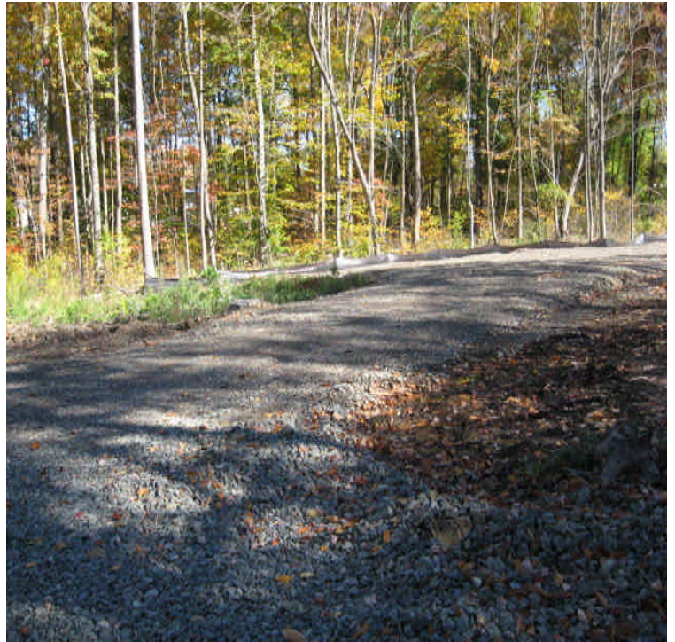
View of a pull site installed upgradient from wetlands near the contractor receiving yard. Controls were installed.
