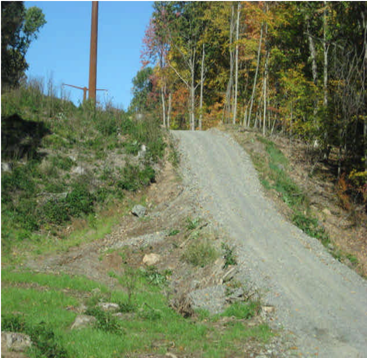
Minor erosion noted along the access road at the steep slope off Black Walnut Drive.
