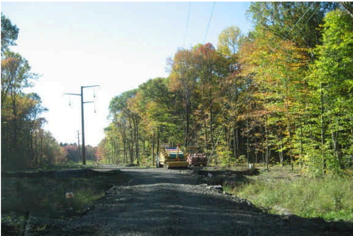
A view of the line pulling equipment and new pull sites installed upgradient from wetlands near the contractor receiving yard.
