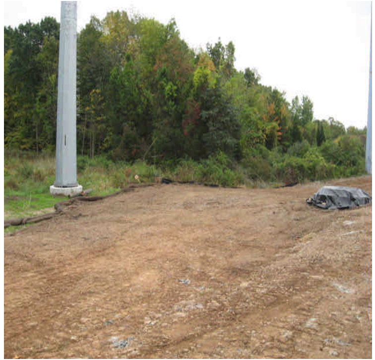
Carpenter Ln (near Beseck): Foundation installed upgradient from wetlands. Some sediment accumulation was noted in the wetlands despite controls in place.
