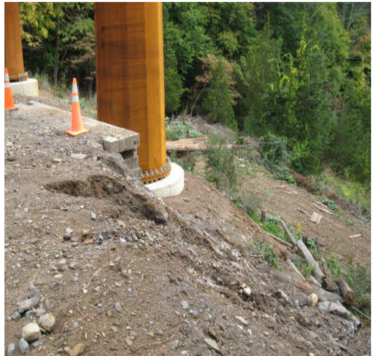
Black Walnut Drive: An eroded washout was present on the pad slope upgradient from Ball Brook. Repair and stabilize; consider using an erosion control blanket if appropriate.
