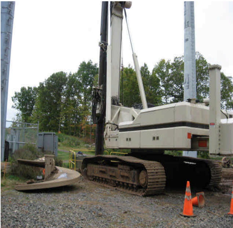
Behind the PBA: View of foundation drilling. The work area was stable and wetlands are not immediately adjacent.
