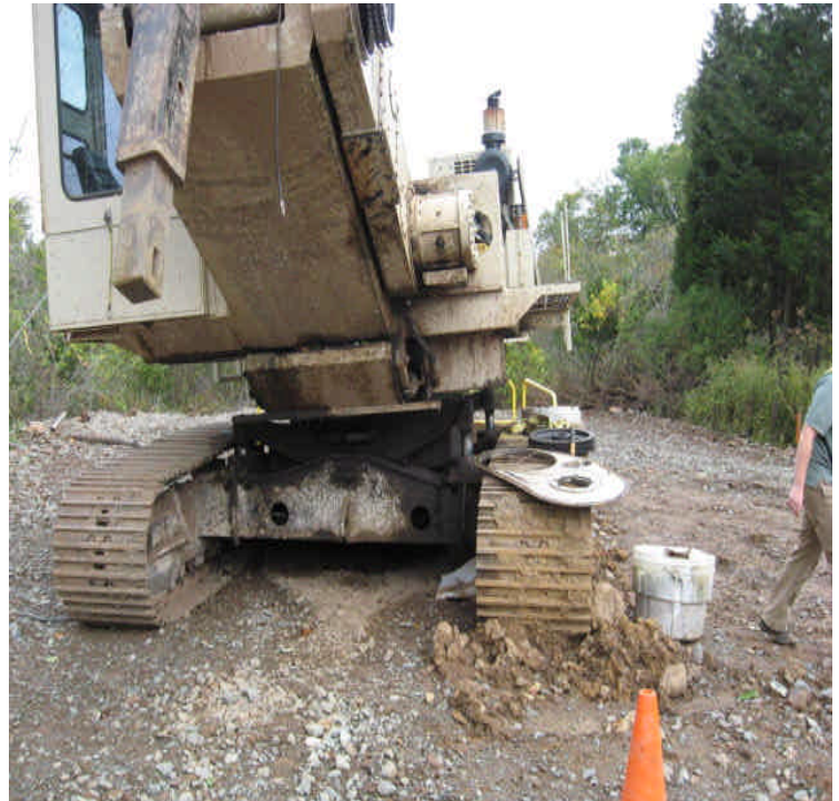
North of High Hill Rd: Broken equipment present near the wetland boundary. Repair and remove as soon as possible. Also, remove any affected soil.
