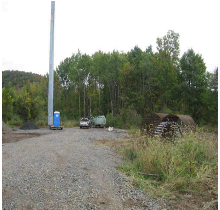
South of East Main St: Air drilling for the next foundation. A sanitary facility was located upgradient from a wetland.
