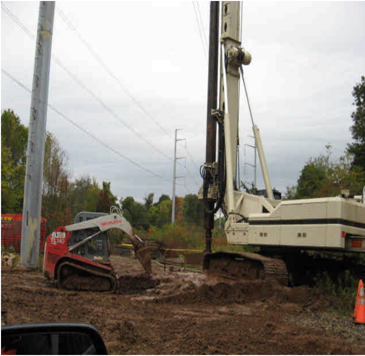
South of High Hill Rd: Drilling within the wetland was underway. Sediment/spoil is being removed as it is generated.
