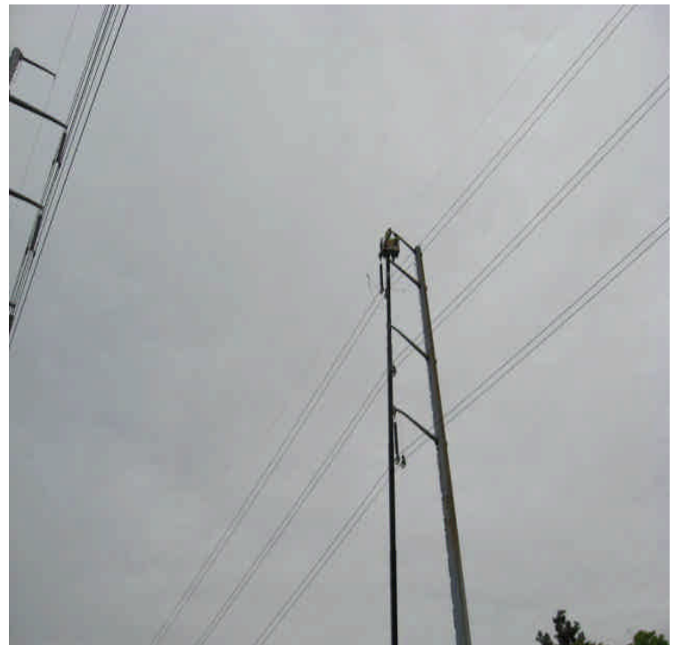
E. Meriden SS: Line work underway. Crews were pulling lines from E. Meriden SS to Beseck SS.
