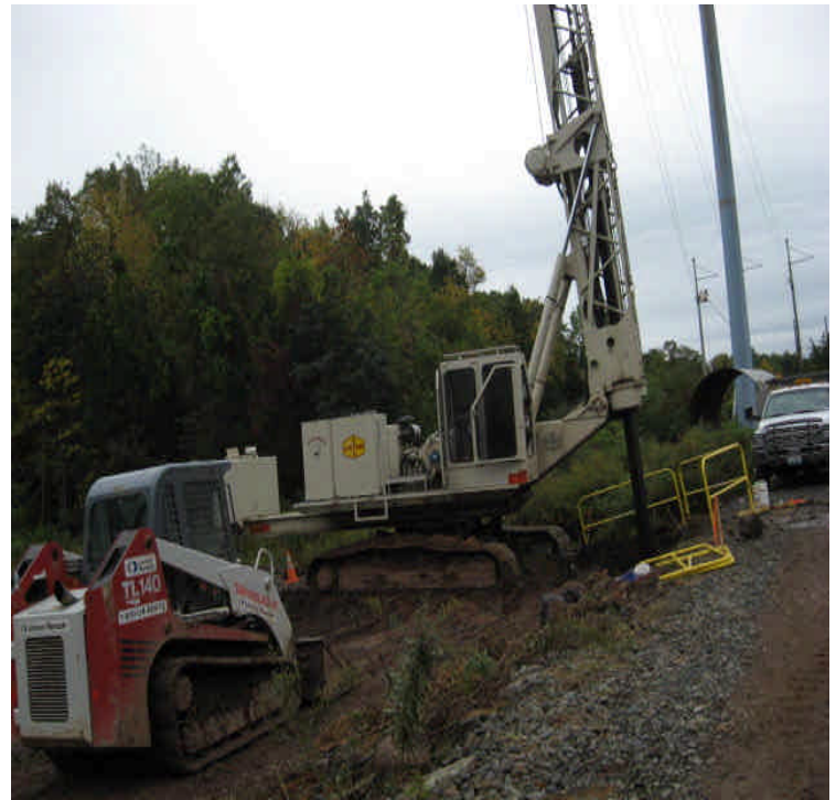
Carpenter Ln (near Beseck): Foundation drilling is occurring up-gradient from wetlands. Sediment/spoil is being removed as it is generated.
