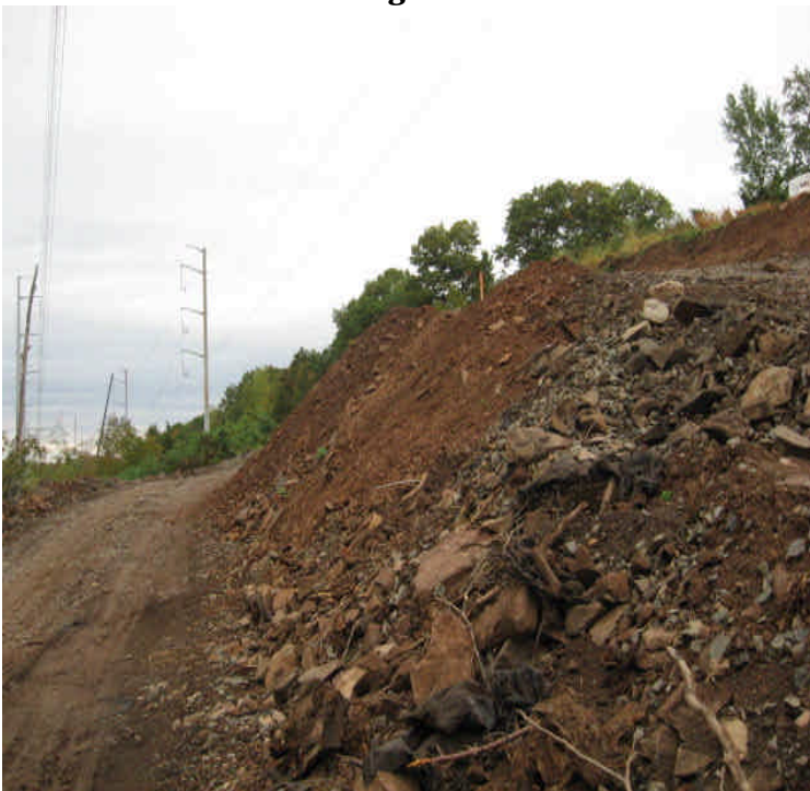
West of E. Meriden SS: Slopes along a new pad site should be seeded and mulched for stabilization. Continue to monitor for run-off; Erosion control blankets may be appropriate due to the steep slope.
