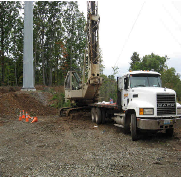
North of High Hill Rd: Broken equipment was noted. Spill controls are in place.
