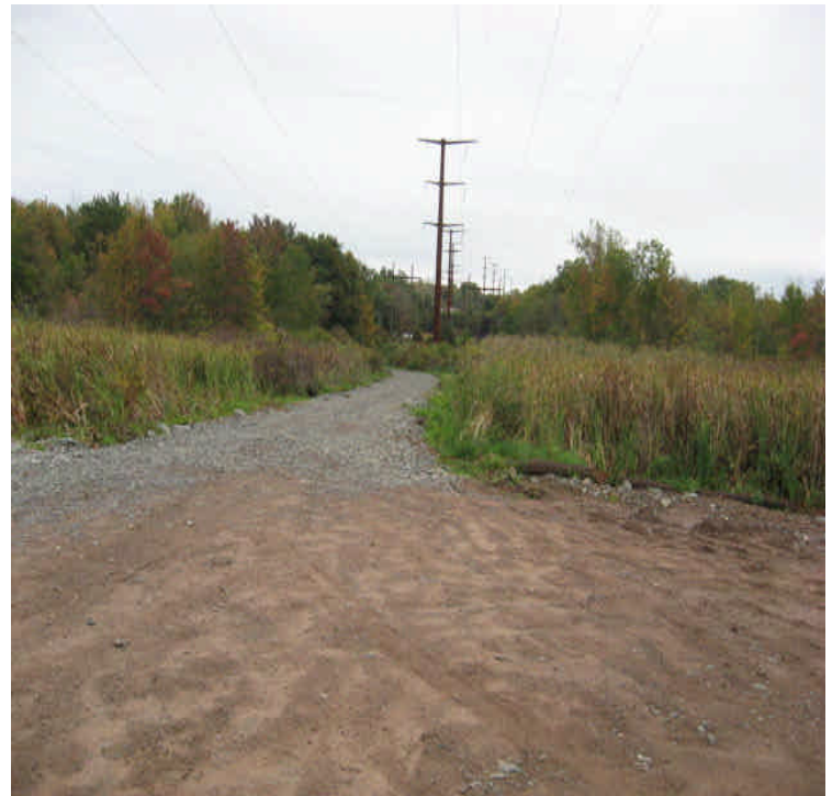
Durham Rd: Sediment migration and accumulation was occurring over the access road and pad within the wetland.
