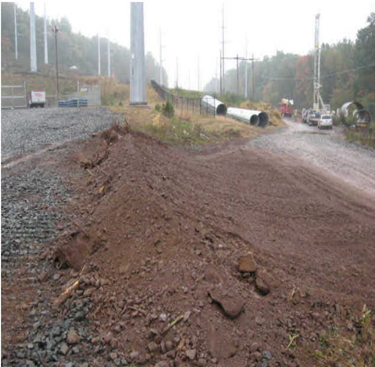
Beseck SS: The original ROW access off Carpenter Ln. was upgraded and is now in use. The constructed access between Beseck and the ROW has now been blocked off. Beseck and 1A contractors should work to stabilize the area with vegetative cover as soon as feasible.
