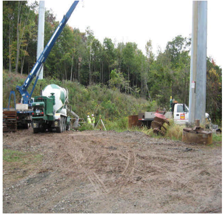
North of High Hill Rd: Crews were pouring concrete at the time of the inspection.
