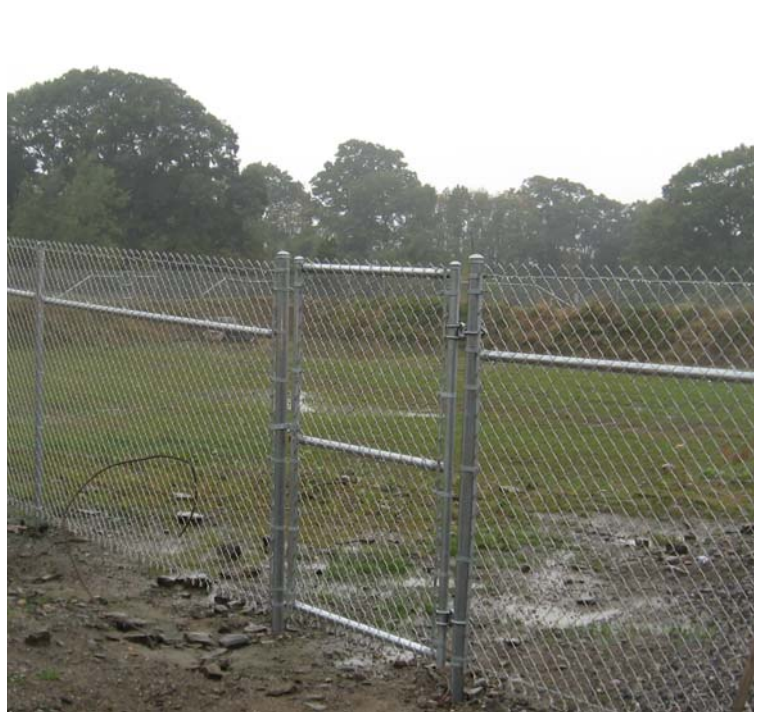
A view of the stormwater detention basin located along the southern site boundary. Increased grass growth was noted here.
