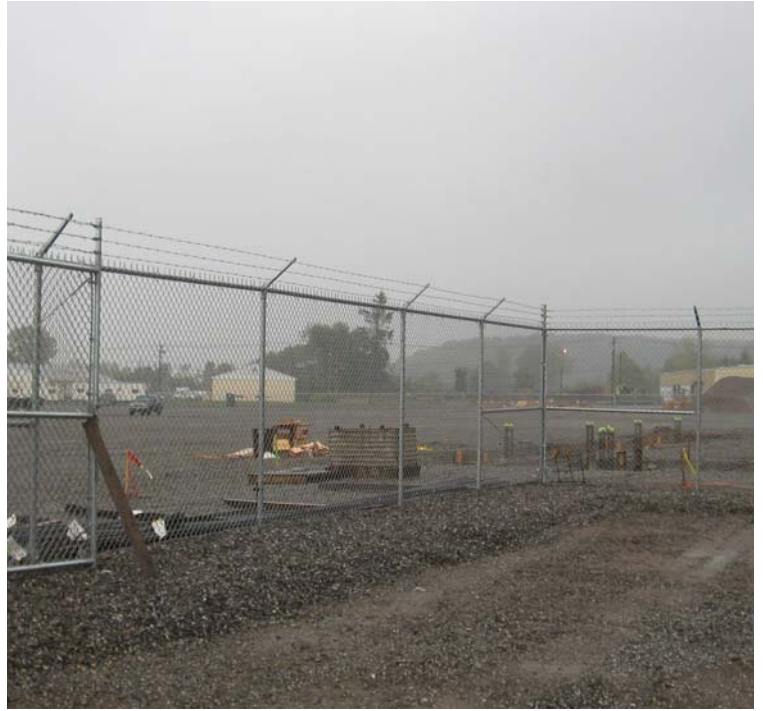
An additional view of the active work at the East Devon Substation.
