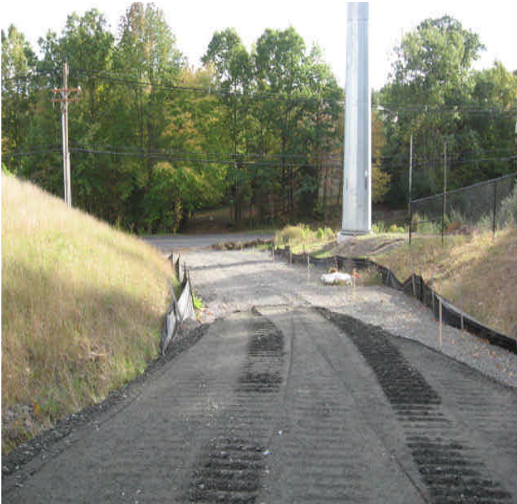
Road base was installed at final grade along the western access road.
