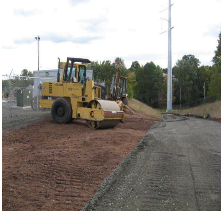
View of the final grading of the western access road in preparation for paving. Soil stockpiles had been used and silt fence controls were removed.
