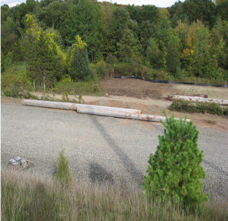
The constructed entrance between BSS and the ROW has been blocked off and graded to prepare for paving the eastern access drive to the station.
