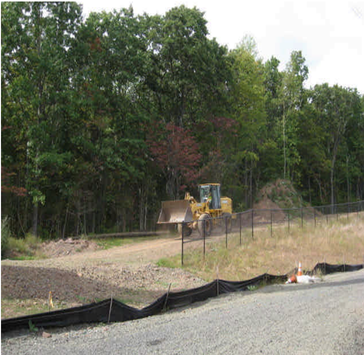
1A contractors were removing the soil stockpile at the old western site entrance, as this is currently an area under their responsibility.
