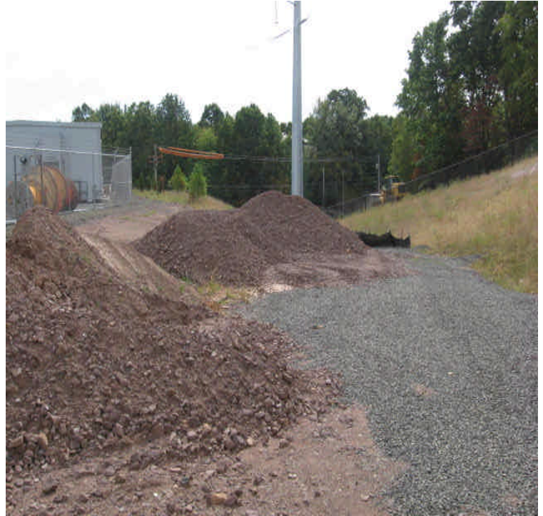
View of the stockpiles and small washouts/eroded channels at the western access drive. Silt fence remains in place across the entrance.
