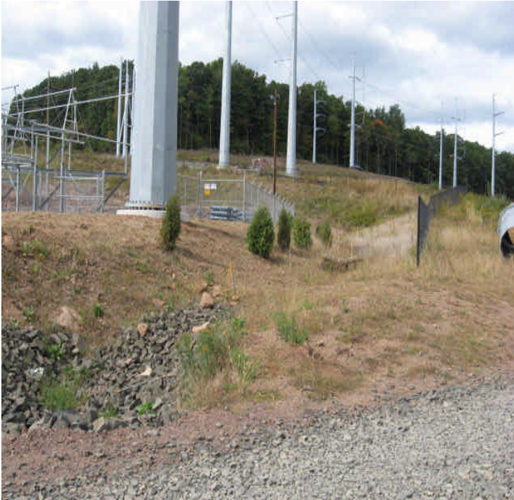
View along the eastern access road. Continue to seed and promote vegetative cover on any bare soil including the recently filled channel.
