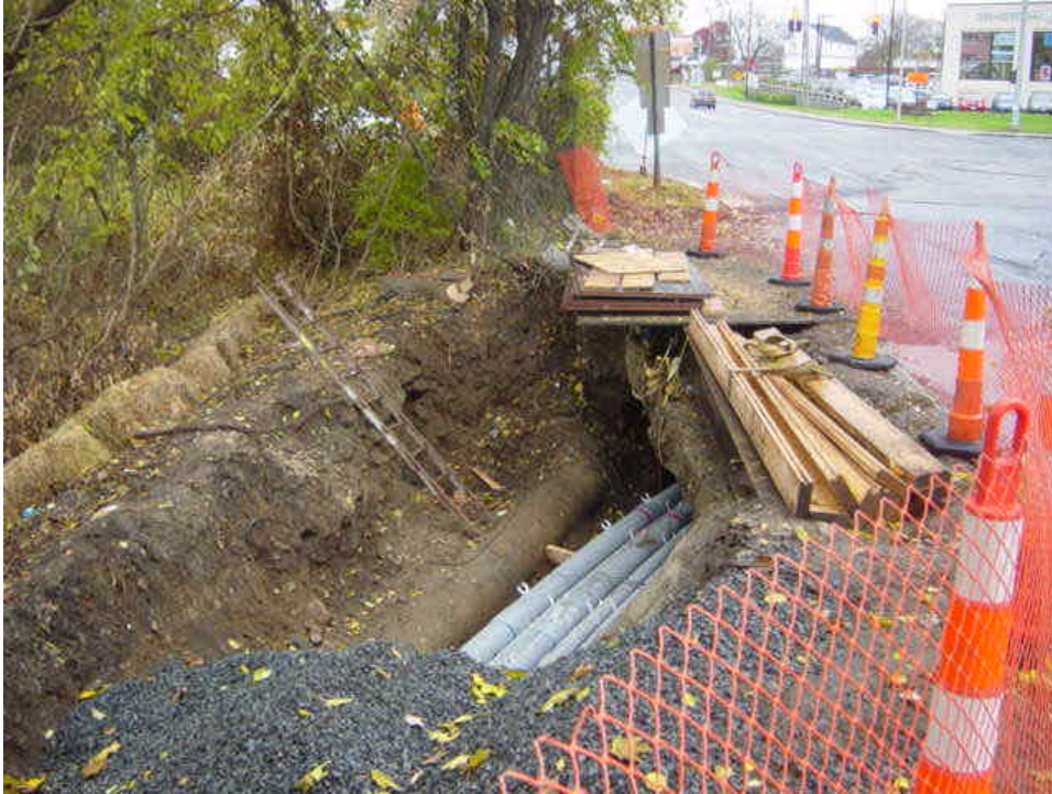
Trench work continues near sta. #16-18 along a fairly steep slope. Haybales remain in place downgradient from the work area along the adjacent slope.
