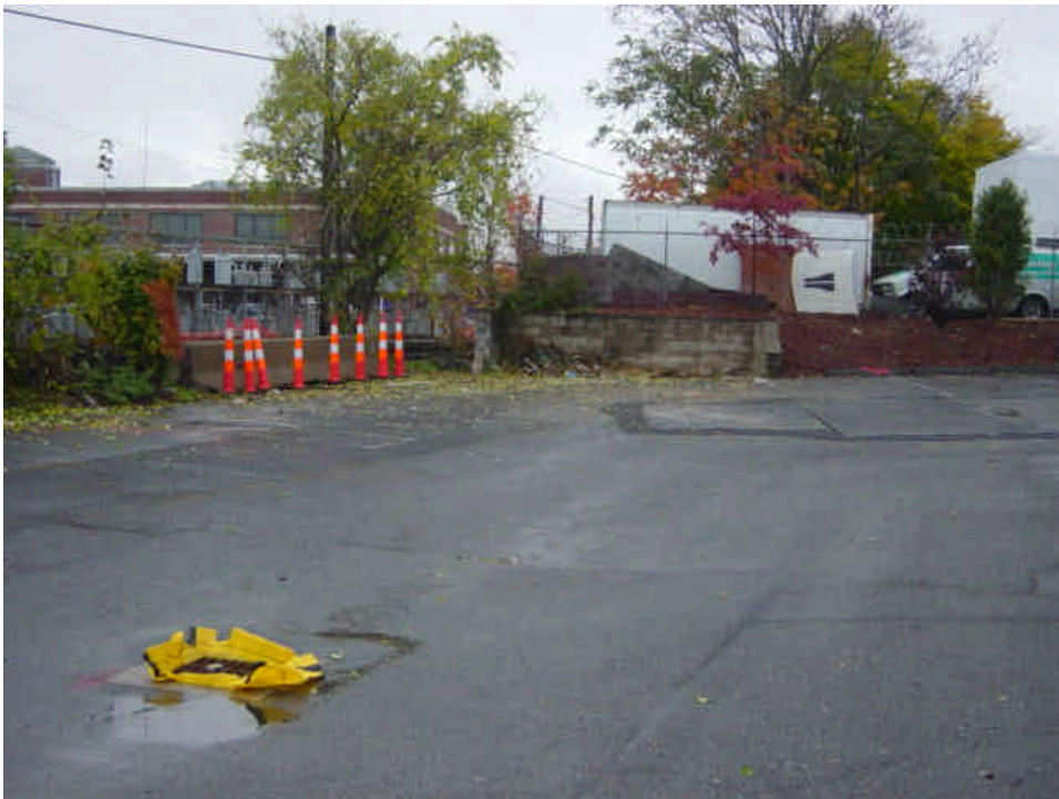
Steel plates are in place over the jack and bore receiving shaft near sta. # 29. The downgradient catch basin has been protected.
