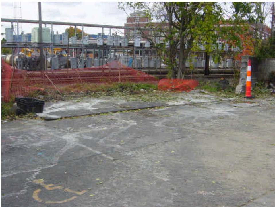
Slurry residue and concrete were cleaned from the paved areas surrounding the work site near sta. # 29. However, the downgradient catch basin still did not have controls in place.
