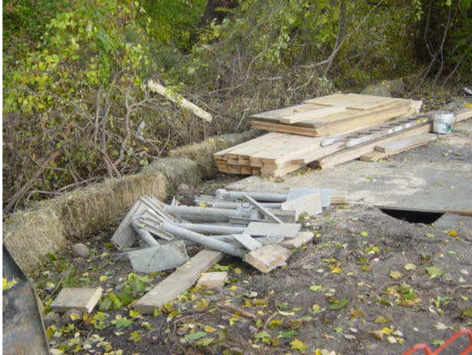
Clearing work has begun near sta. #16-18 along a fairly steep slope. Hay bales have been installed downgradient from the work area along the adjacent slope.
