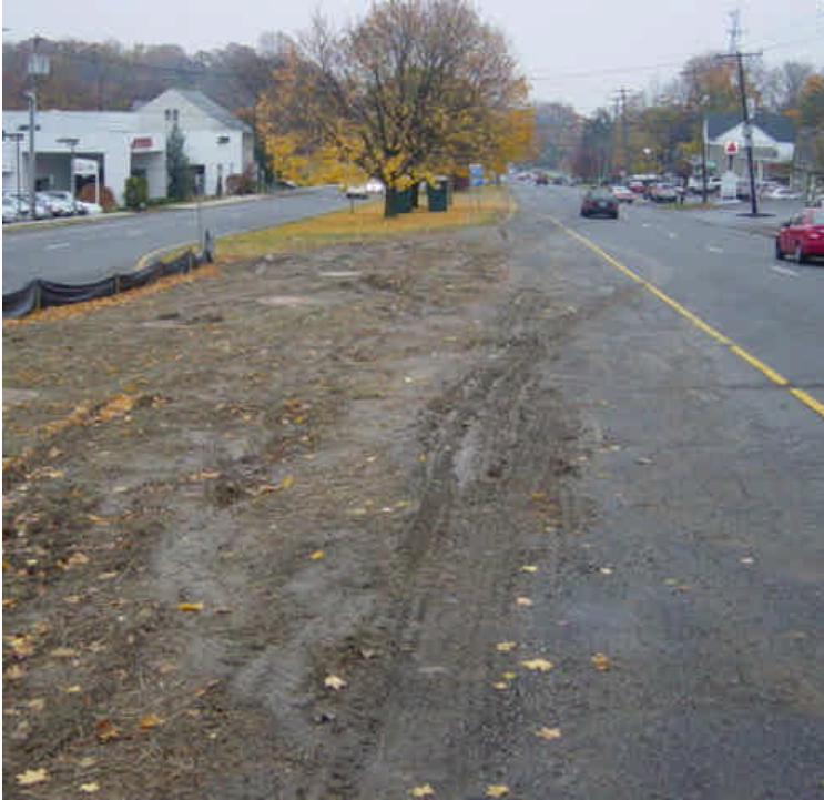
Minor tracking was observed near sta. #316-318. Hay mulch was previously applied over the exposed soils, but the area should be refreshed so there is a sufficient layer of cover for the winter months.
