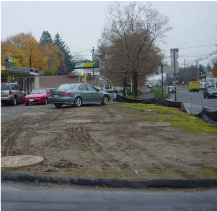
Vehicles continue to park on the seeded areas/exposed soils near sta. #334 (vault #20). Minor tracking was observed in the parking lot. Refresh with mulch cover sufficient for the winter months. Work out a parking plan with the landowner.
