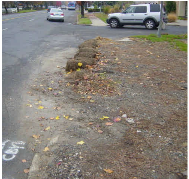
Minor sediment accumulation was observed along the shoulder of the roadway near sta. #381-383 (vault #23). The accumulation was heavier in areas where the curbing has deteriorated. Hay bales are providing some control, but the bales are also deteriorating.
