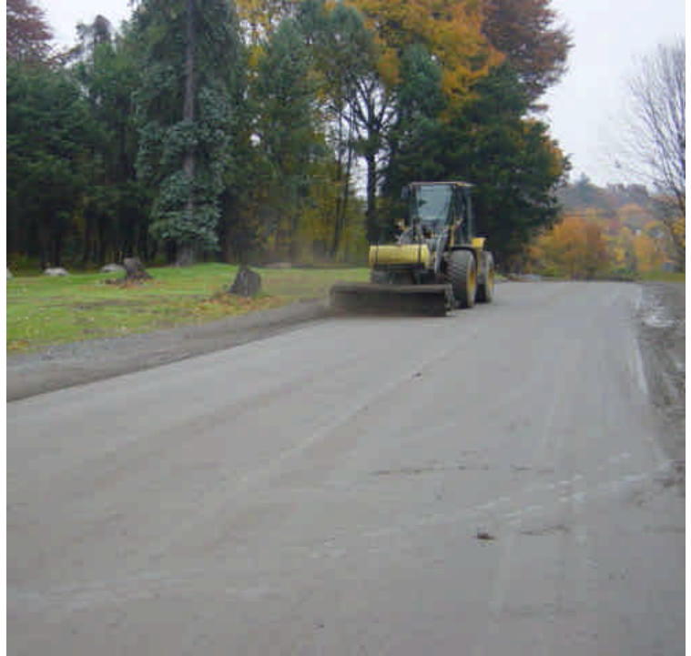
Minor tracking was observed along the access road to the Sherwood Island lay-down yard. Crews were observed sweeping the access road at the time of the inspection.
