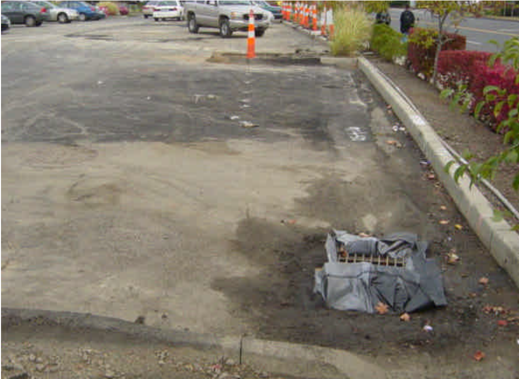
Steel plates are in place over the exposed trench near sta. #96, as tie-in work continues at vault #6. The silt sack in the catch basin has been replaced but heavy sediment remains in the parking lot area following the water ponding here last week.
