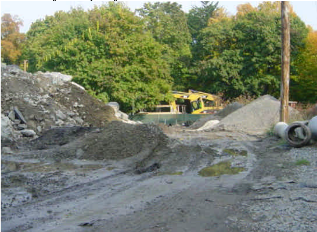
Stockpile of debris material in the Sherwood Island lay-down yard is growing very large. Saw cutting slurry was dumped near the edge of the debris pile on the access road within the yard, increasing the potential for tracking.
