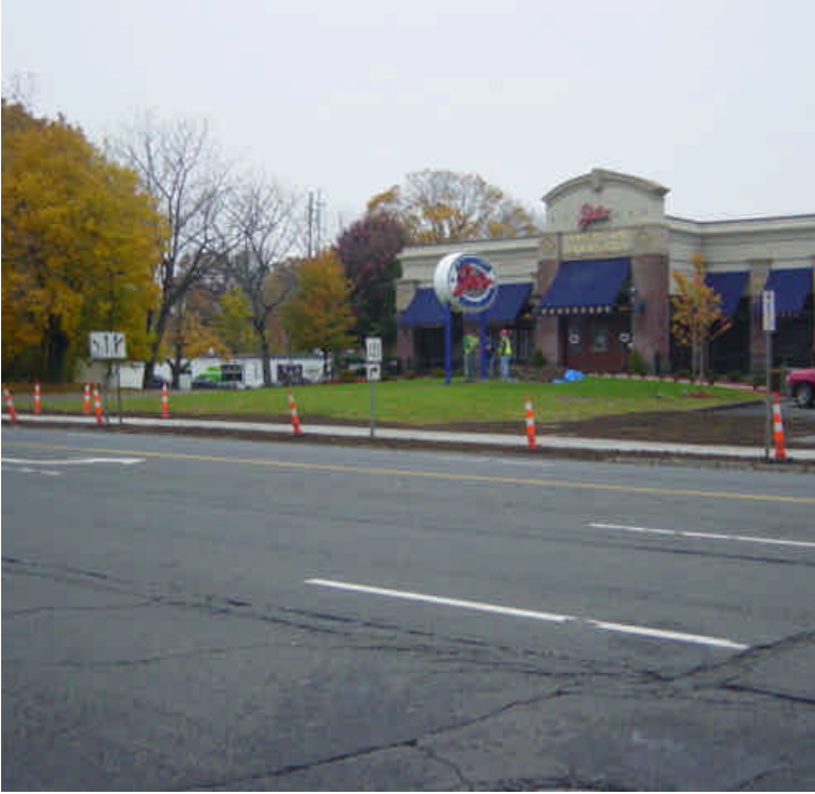
Permanent restoration work is underway near sta. #596 (vault #36) as a new sidewalk has been installed. Ensure that any landscaped areas are appropriately stabilized.
