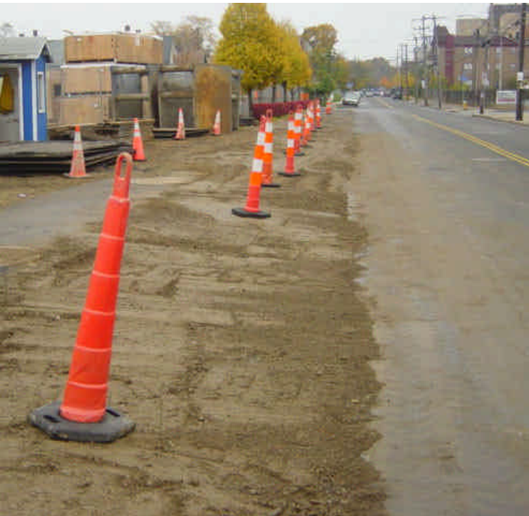
Area between sta. #801-803 has been backfilled. Exposed soils need to be stabilized. Minor sediment tracking was observed along the shoulder of the roadway.
