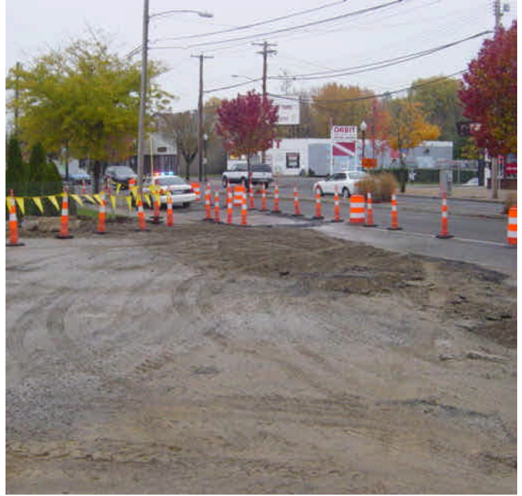
A large area of exposed soil is adjacent to the work area near sta. #649-650. Minor tracking was observed at the entrance/exit of the work area.
