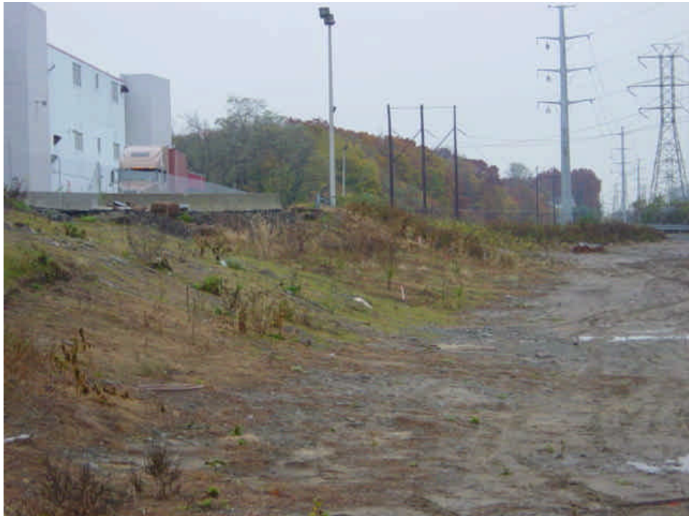
The slope near sta. #1080 is temporarily stabilized with vegetation. Final restoration is still required once an agreement is reached with the adjacent landowner.
