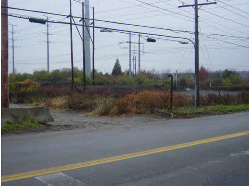
Sediment tracking continues near the entrance to the right-of-way near sta. #1080. Tracking does not appear to be associated with this portion of the project. The stone construction entrance has area has deteriorated and needs to be refreshed with new stone. This responsibility should be coordinated with overhead contractors. See the 2B report.
