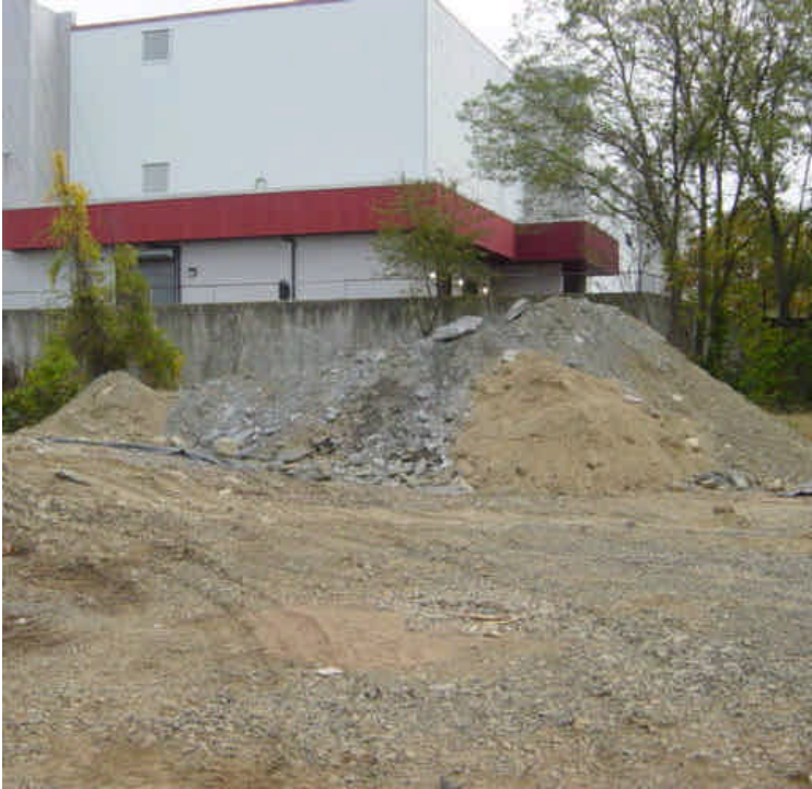
Work noted on the overhead lines along the cross country section between sta. #1051 to #1080 which overlaps the Segment 3 route. Several stockpiles were noted along the ROW, but erosion controls were not provided
