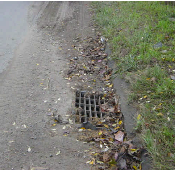
Tracking was evident along Caswell Street, but does not appear to be associated with this portion of the project. The catch basin was protected previously, but the silt sack is torn and in need of repair.
