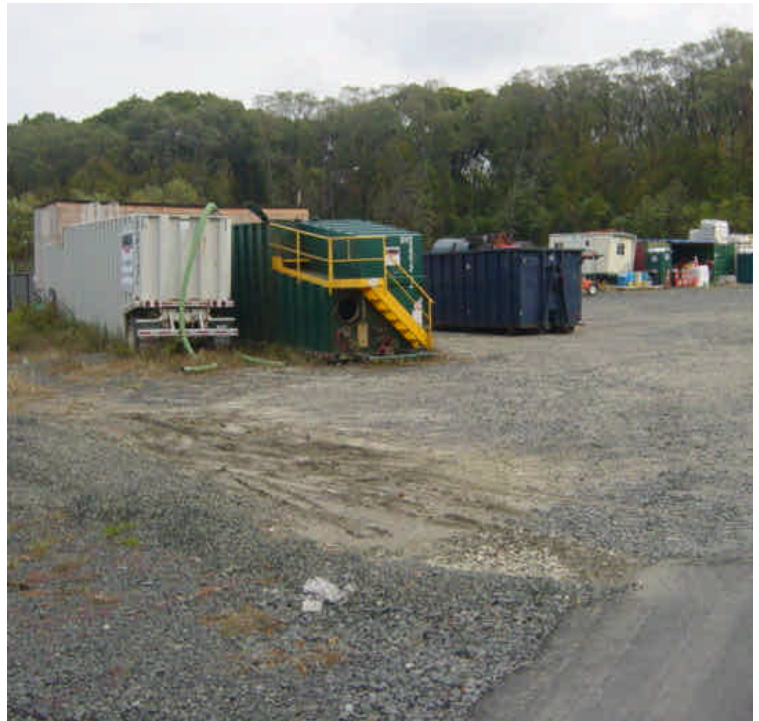
Shelland St. laydown yard remains inactive as work has shifted to other areas of the project. Perimeter controls continue to function, but require maintenance when work returns to this area.
