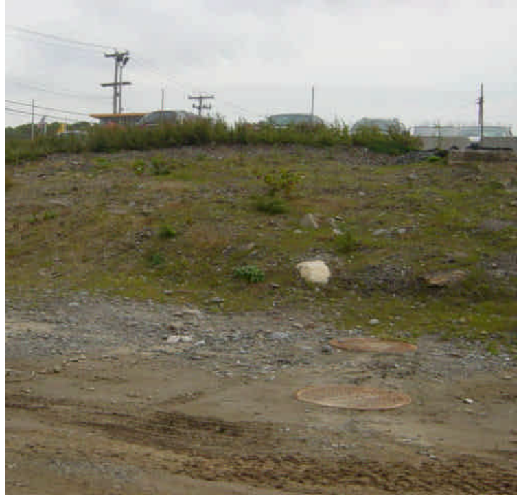
The exposed soil along the slope near sta. #1080 has re-vegetated naturally (approximately 75% coverage). The slope will be fully restored in the future. A plan is being worked out with the landowner.
