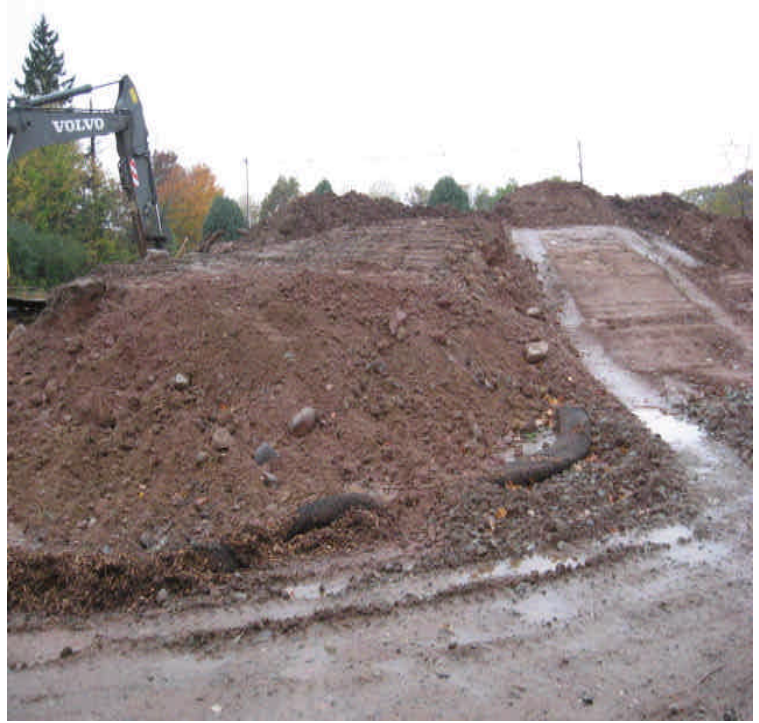
Pond Hill Dr: Soil stockpiles from other sites are being stored here. Controls have been overwhelmed by sediment and should be replaced or reinforced.
