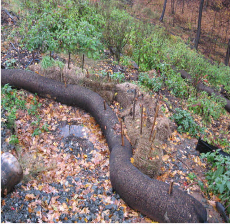
Harrison: Controls are in place across the eroded gully leading from the drainage basin. They are functioning well but the gully should still be repaired/restored.
