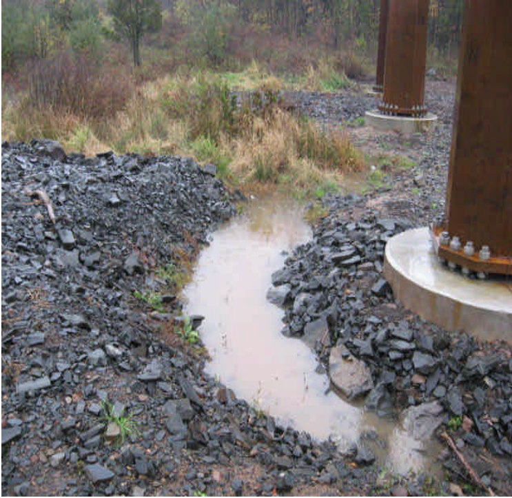
Carpenter Ln: Turbid water was observed within the wetlands during a rain event.
