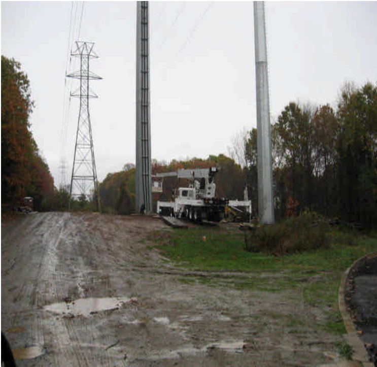
Old Farms Road: Turbid run-off was noted at a disturbed/exposed area during a rain event.
