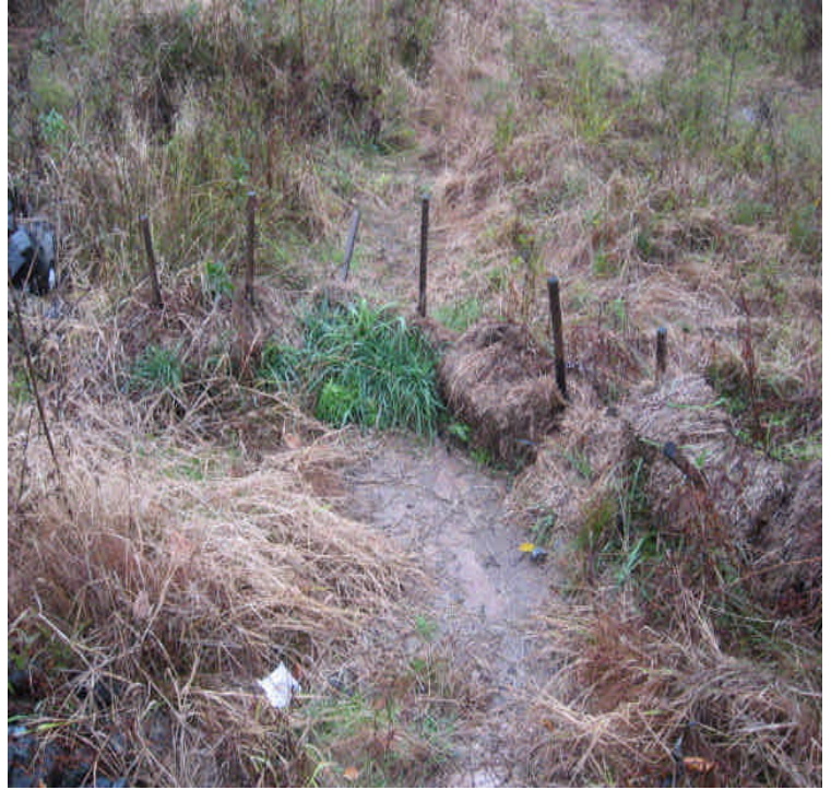
Carpenter Ln: Deteriorating controls and sediment accumulation was noted at the wetland outlet. This area still receives turbid run-off during rain events.
