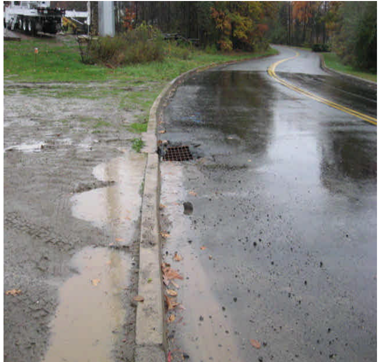
Old Farms Rd: Turbid run-off flowing from the ROW and into a catch basin in the roadway. This water then flows off-site into wetlands.
