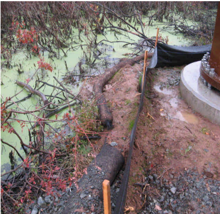
Tamarack Swamp Rd: The silt fence remains in place but the sediment that had been pushed beyond the original controls should be removed carefully.
