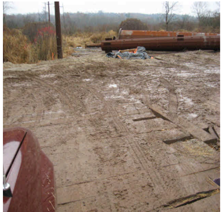
Durham Rd Golf Course: Foundation drilling complete. Sediment from the drilling has been removed from the timber mats.
