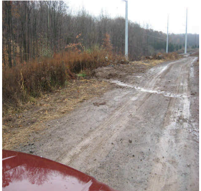
Beseck SS: Water bars have been installed to divert stormwater to stable areas.
