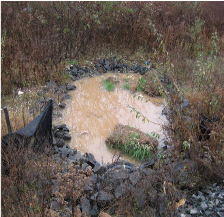
Beseck SS: Turbid water from the access road was overflowing from the sediment trap. Wetlands are located to the east.
