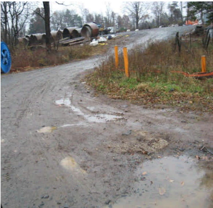
Contractor Receiving Yard: Deteriorated controls remain along the access drive, upgradient from the wetland.
