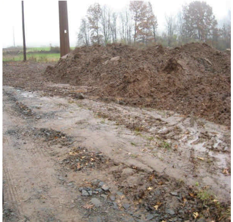
Little Lane: Stockpiles from other sites are being stored in the uplands. A slurry pit has been filled in. Add controls as needed around the stockpile if it is to remain.
