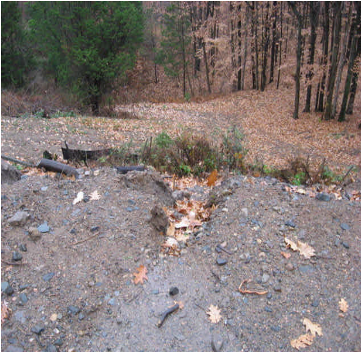
Black Walnut Dr: Silt fence remains in place upgradient from Ball Brook at the base of the washouts. Monitor silt fence but address the problem at the source. Repair the gullies and re-stabilize the slope, especially as work activities are not returning
