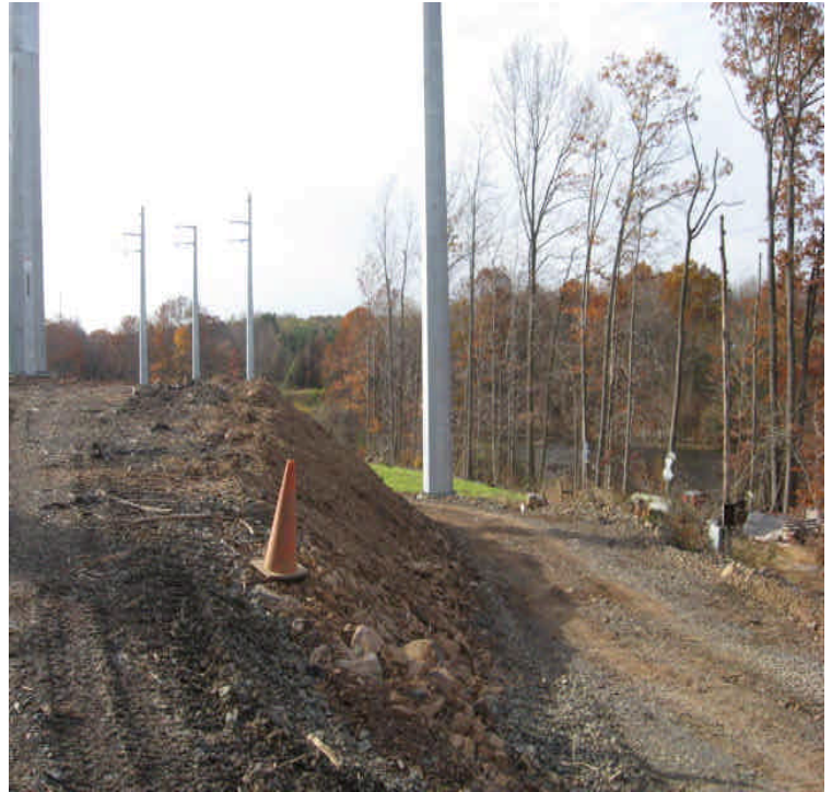
East Meriden SS: The steeply sloped edge of a pad site in this area has been mulched.
