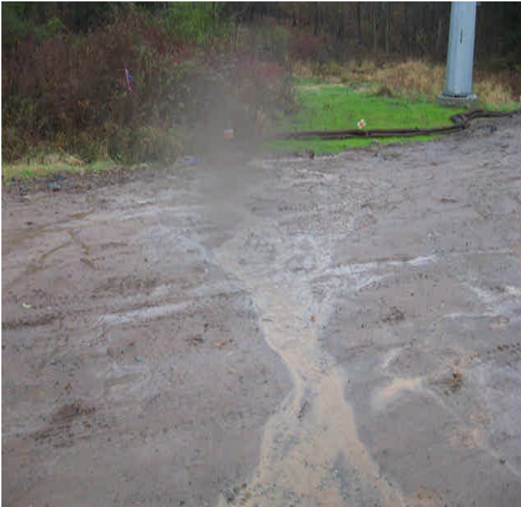
N.E. Beseck SS: Turbid water flowing into wetlands from the access road. Reinforce controls as needed.
