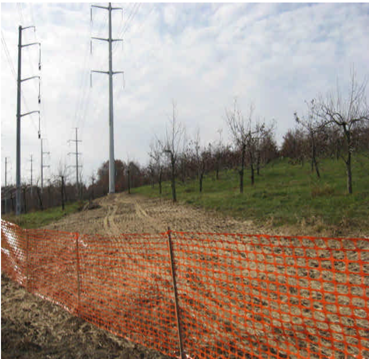
East Meriden SS: Several exposed areas have been mulched and seeded and cordoned off from vehicle access.
