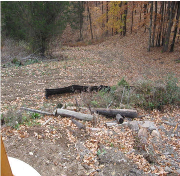
Black Walnut Dr: Silt fence installed upgradient from Ball Brook at the base of the washouts. Monitor silt fence but ultimately address the problem at the source. Repair the gullies and re-stabilize the slope, especially as work activities are not returning.
