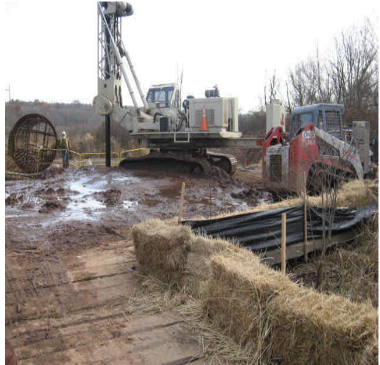
Durham Rd Golf Course: Sediment pile noted on timber mats from foundation drilling. Controls are in place and should be monitored.
