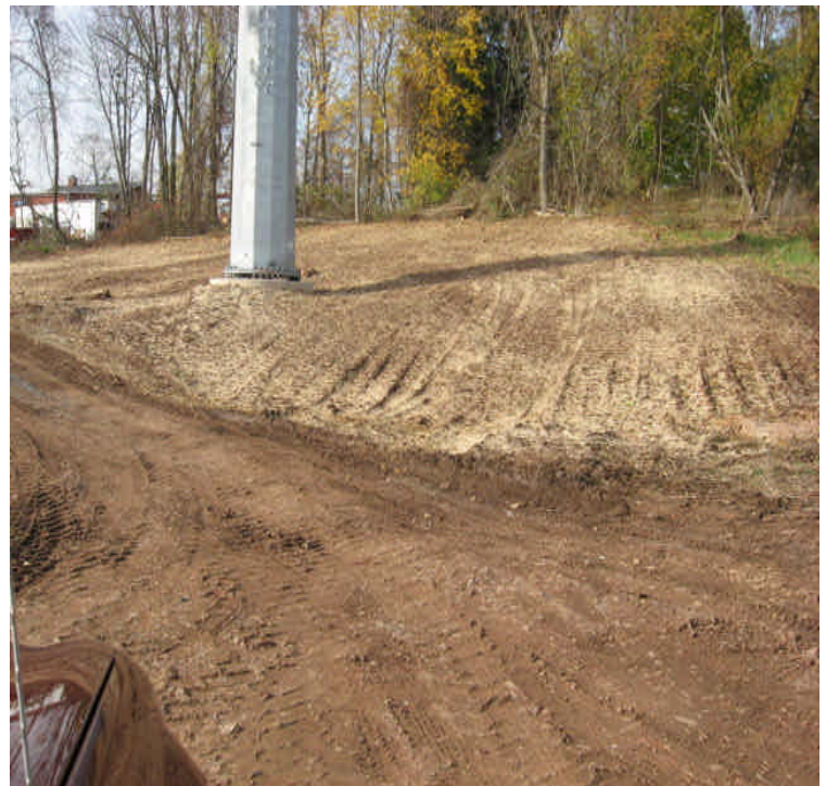
North of East Main St: Exposed area located upgradient from the wetlands has been mulched and seeded. Monitor to ensure that the amount of mulch cover is appropriate for stabilization throughout the winter.
