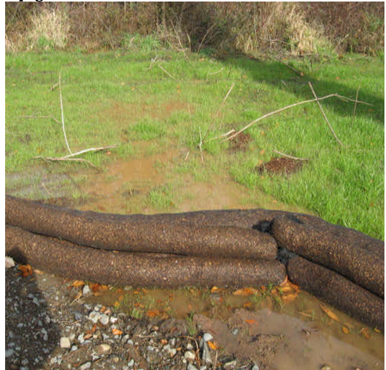
East of Besock SS: Following a rain event, turbid water was flowing from the access road and pad site, into the wetland here. Determine how to reinforce controls and make them more effective.
