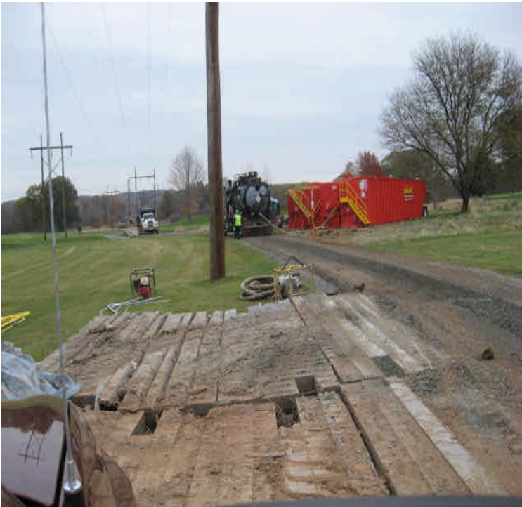
Durham Rd Golf Course: Dewatering during foundation drilling. Frac tanks were being used.
