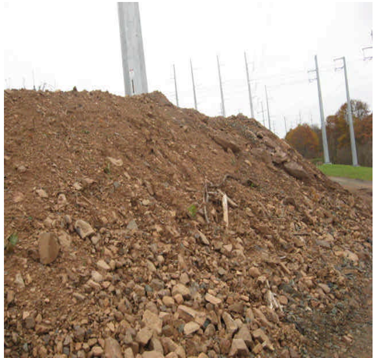
East Meriden SS: The steeply sloped edge of a pad site needs controls/stabilization.
