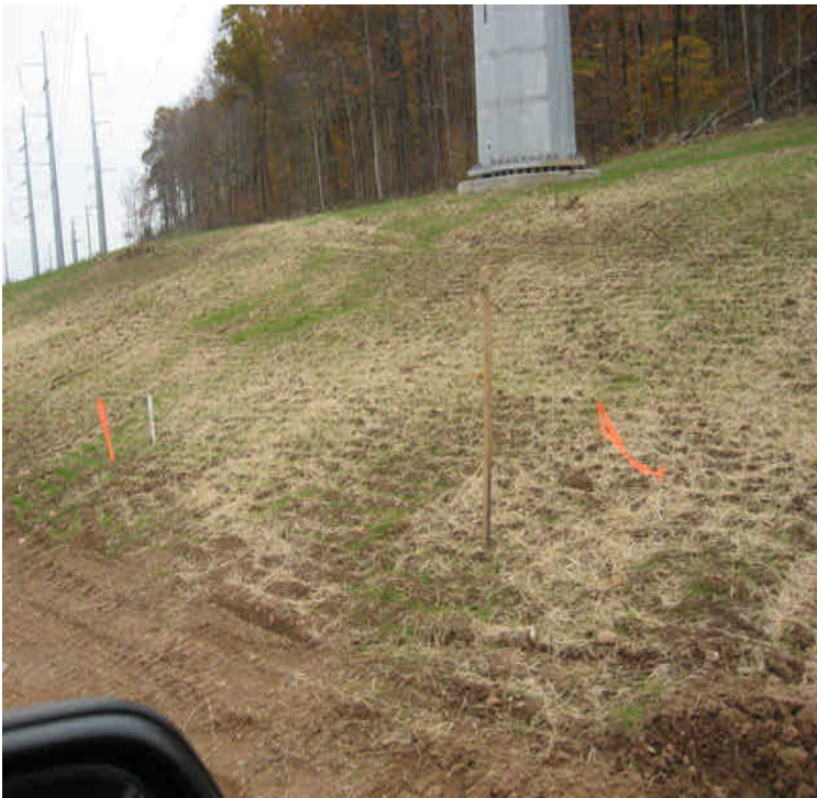
N. Beseck SS: Mulched and seeded areas located at recent pad sites are growing some grass cover. Continue to monitor into the winter for stabilization.
