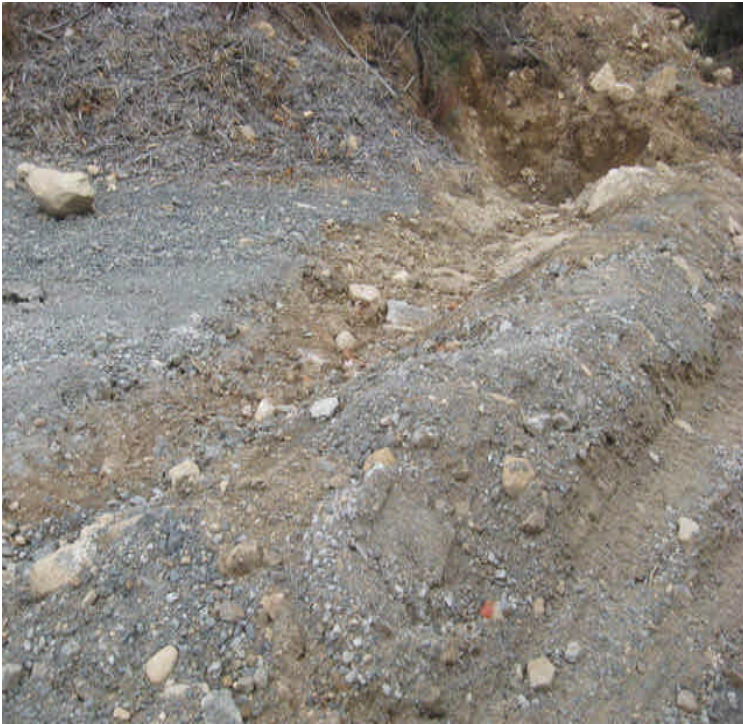
East of Rte. 9: Drainage ditches were installed along the access road. Ensure that run-off is directed to stabilized/vegetated areas and that the swale itself is stable.
