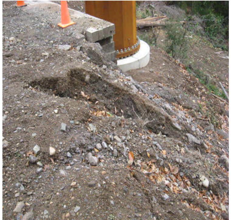
Black Walnut Dr: Ruts and erosion noted along a steep slope on the last pad site upgradient from Ball Brook. Regrade and stabilize; consider adding an erosion control blanket due to the slope grade.
