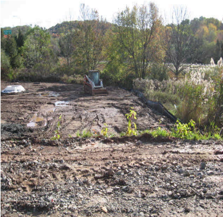
North of E. Main St: Foundation drilling is complete. Controls are in place. Continue to monitor carefully. Stabilize and restore disturbed areas as soon as possible, especially adjacent to the wetlands.
