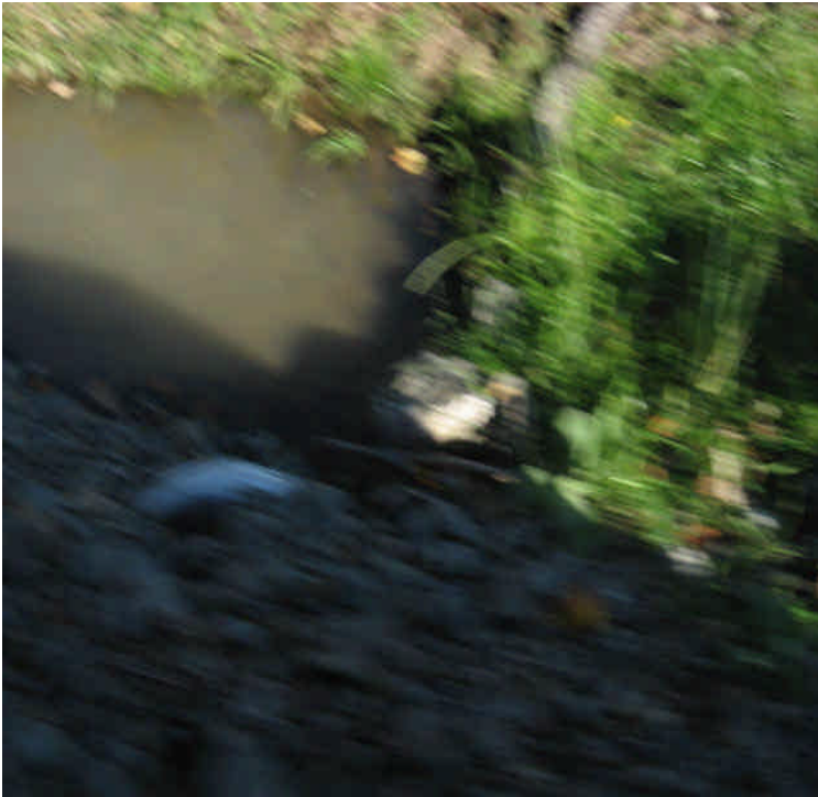
Shumpike Rd.: Turbid water noted at a culvert under the access road. Run-off from the sloped access road is resulting in the turbid water.
