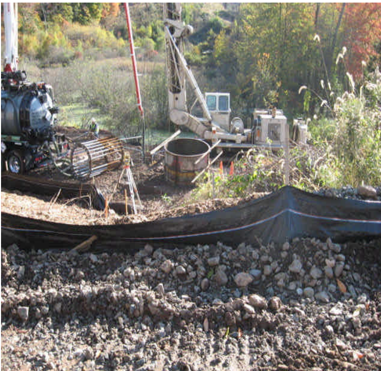
Black Pond Jct: Foundation installation is underway. Crews were pumping slurry into a settling tank onsite. Controls are in place. Continue to monitor carefully due to wetlands in the area.
