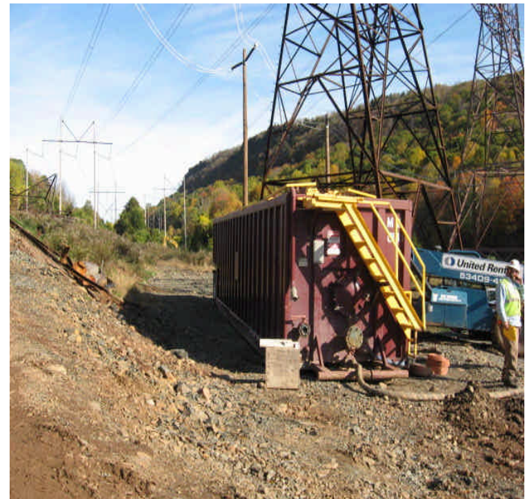
Black Pond Jct: Settling tanks were brought to the site for foundation installation and associated dewatering
