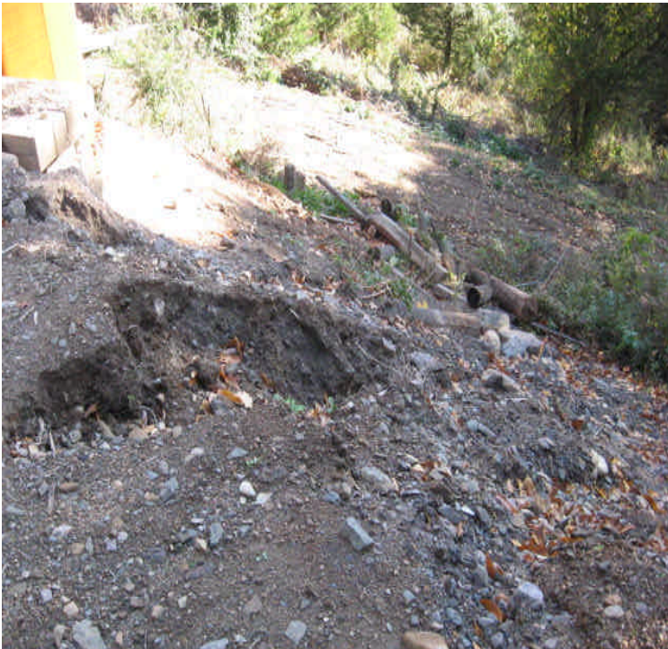
Black Walnut Dr: Ruts and erosion noted along a steep slope on the last pad site upgradient from Ball Brook. Regrade and stabilize; consider adding an erosion control blanket due to the grade.
