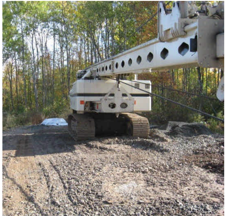
South of E. Main St.: Foundation installation is complete. Controls are needed as a large disturbed area is present upgradient from wetlands. Equipment is also parked upgradient from wetlands.
