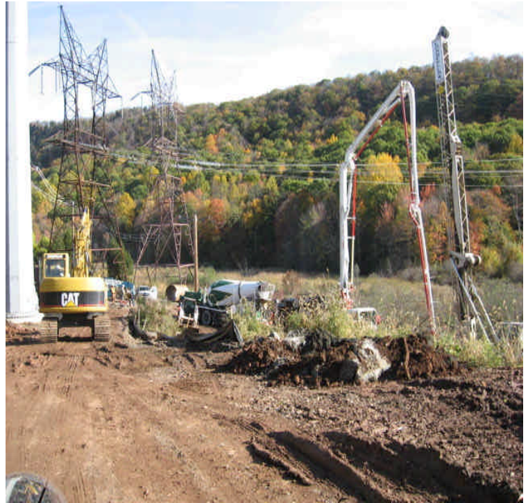
Black Pond Jct: Foundation installation underway. Pump truck and settling tanks were used for dewatering
