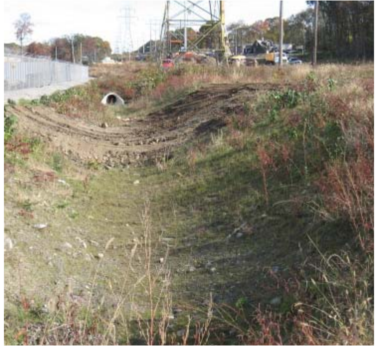
East Devon Substation: Exposed soils were observed within the drainage swale. Temporary stabilization is necessary here.
