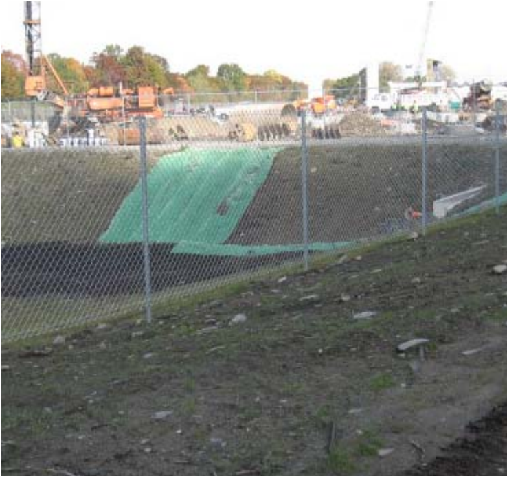
East Devon Substion (Milford): A general view of construction at the substation. Erosion control blankets were being installed along the detention basin slopes.
