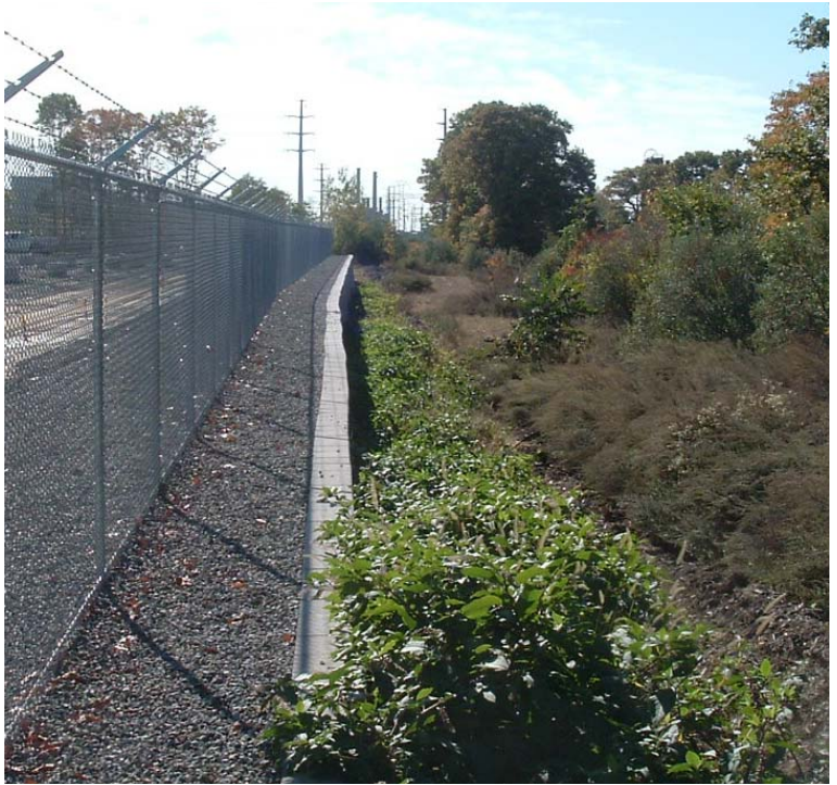
East Devon Substation: A view of the retaining wall located along the western site boundary.
