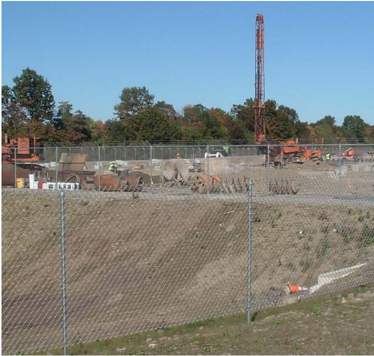
East Devon Substation: A view of the substation from the southern site boundary.
